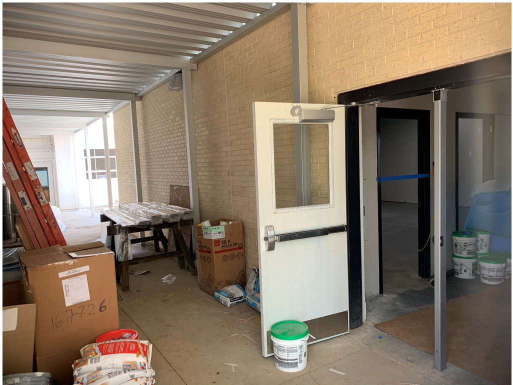
Figure 2 – Rear Exit Corridor; this area needs to be kept clean for egress from main building in case of an evacuation event.
