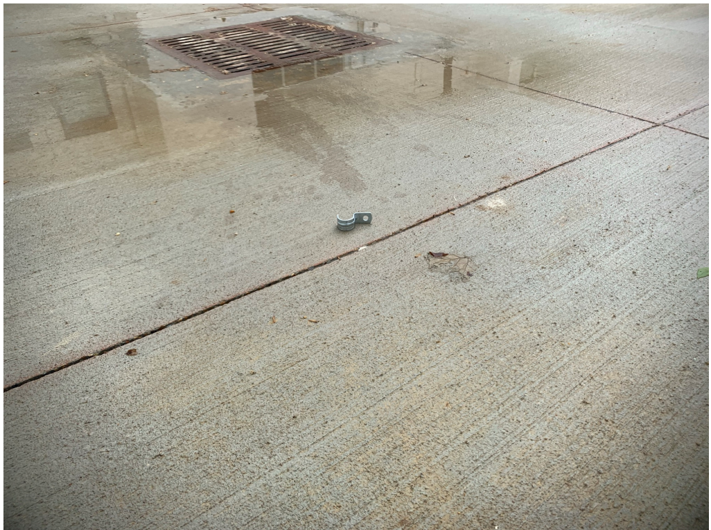
Figure 8 – Standing water around inlet needs correction
