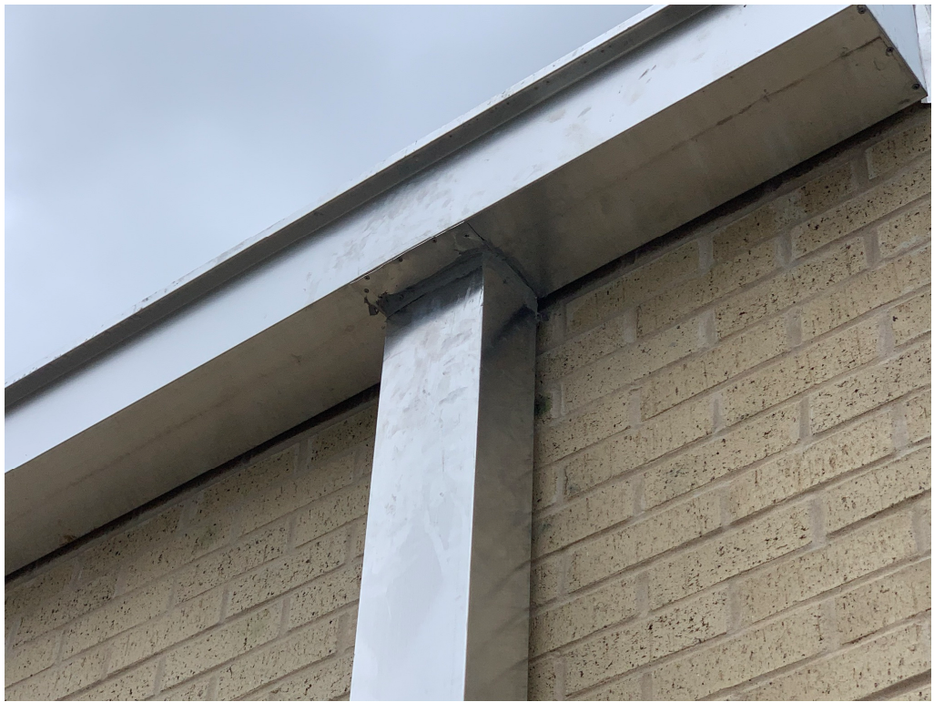
Figure 7 – Sloppy Sealant at Downspouts; are these to be covered with cover plate so that fasteners do not show?
