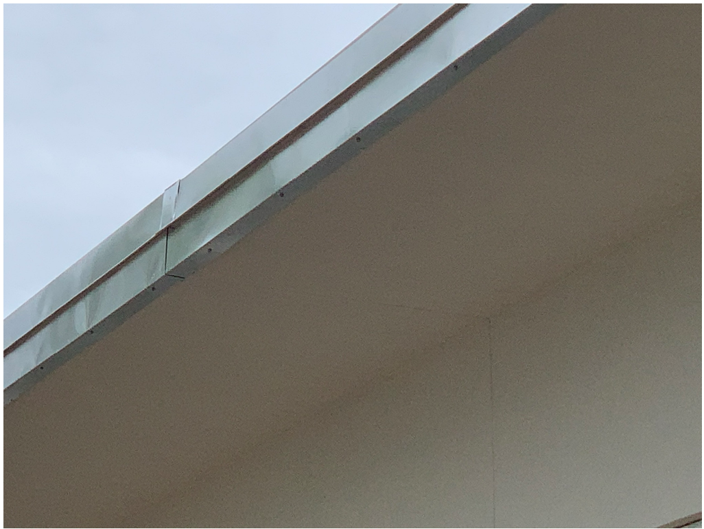
Figure 3 – Is there a finish piece of trim to hide these fasteners and wavy flashing?
