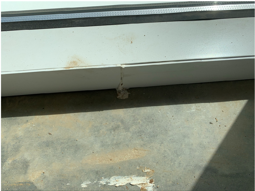
Figure 8 – Caulking & Storefront will need to be corrected any place where not smooth or flush or gaps found between metal trims
