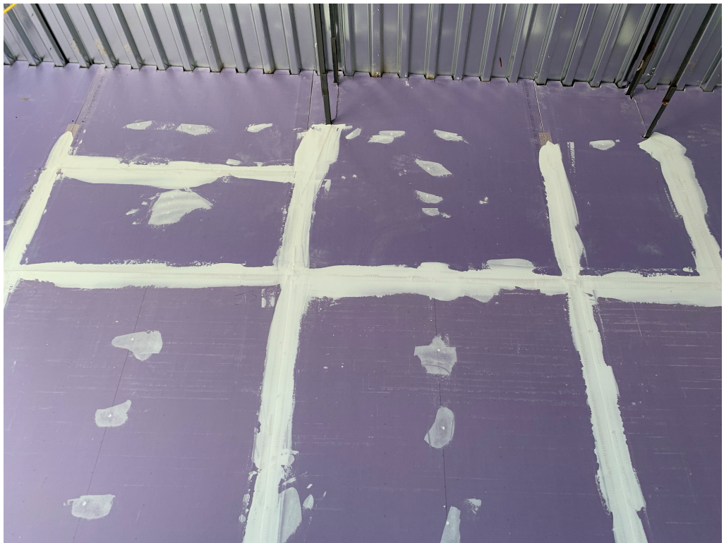
Figure 4 – Some flex noted in walls; contractor to complete drywall installation including perimeter screw pattern at all sheets as well as add kickers in hall as needed
