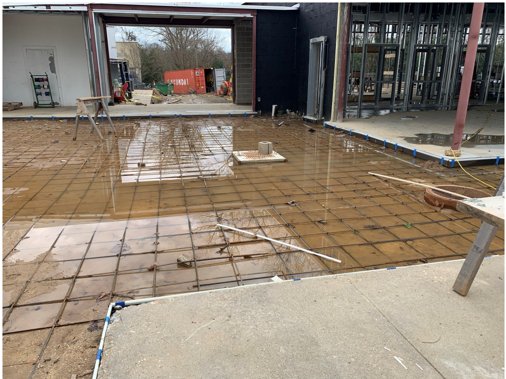
Figure 4 – Drainage Issues at Courtyard
