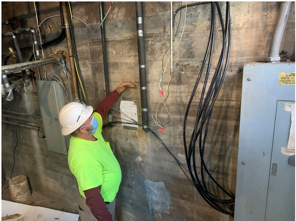
Figure 10 – Plumbing/Electrical Conflict (awaiting resolution)
