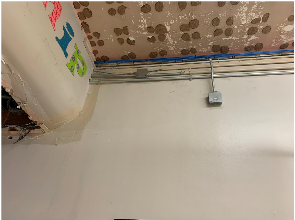
Figure 13 – Conduit Removed from Bulk Head Drop Down at main Hall; This junction box could be re-run above ceiling
