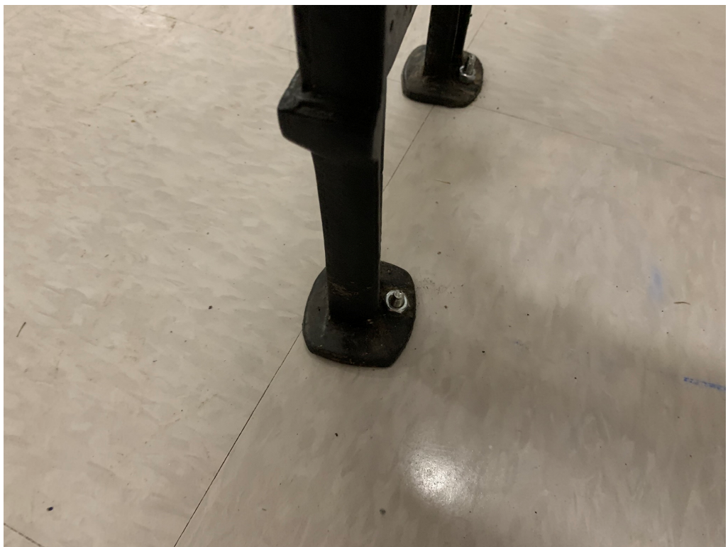
Figure 8 – Concrete Anchors Require some Black Touchup Paint so that they do not stick out
