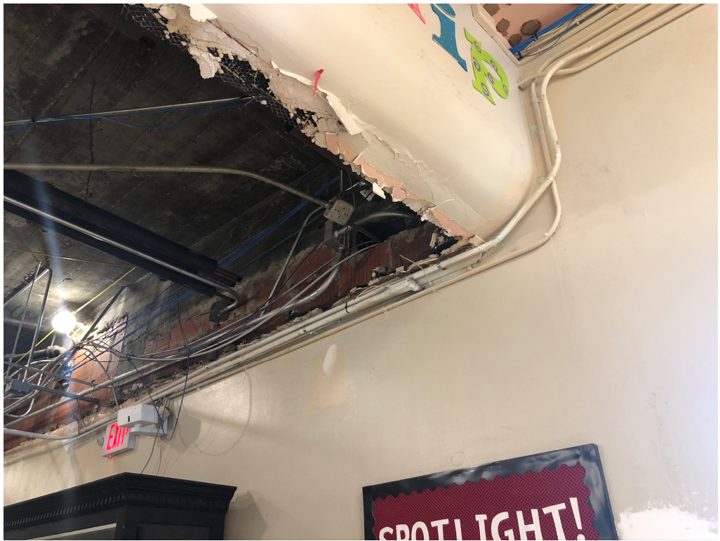
Figure 17 – Camera Connected Through Conduit to be Removed (Camera Needs to be disconnected by School Staff for Contractor to move forward)
