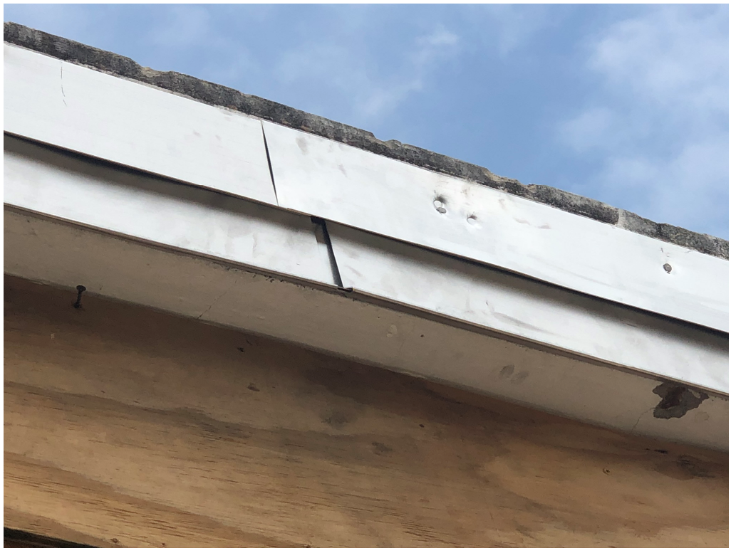
Figure 6 – Nail Pattern Uneven and irregular
