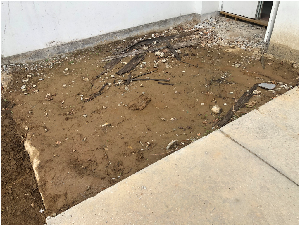
Figure 10 – Demoad Concrete in South Corner of Rear Yard
