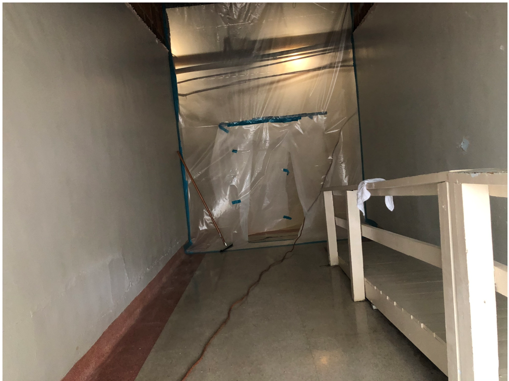
Figure 2 – Secondary Asbestos Plastic Protection
