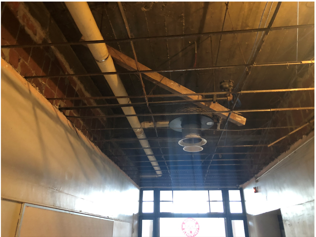
Figure 12 – Existing 4x4 Atop Boiler Pipe to Support Ceiling
