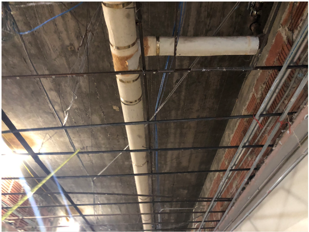
Figure 7 – Pipe prevent duct runs from crossing each other
