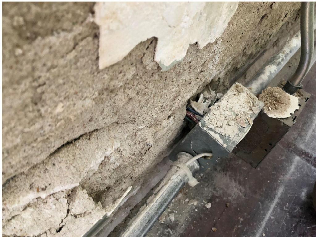
Figure 6 – Wire through wall is not in conduit
