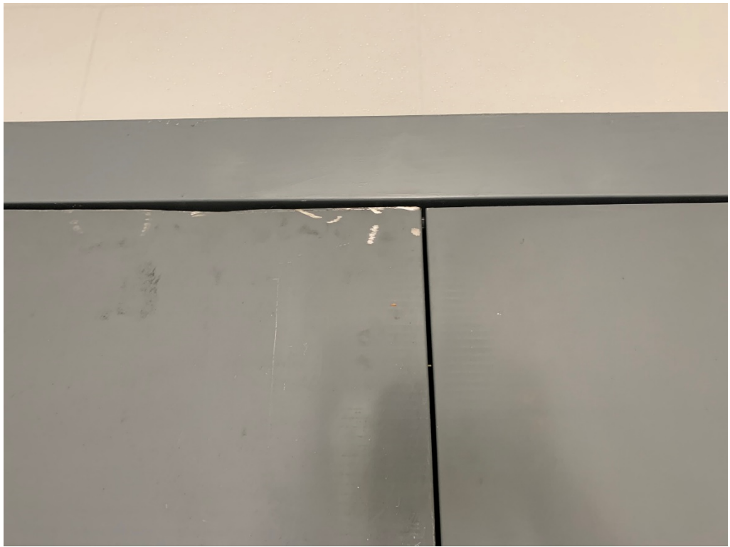
Figure 5 – Top of Door Edge has Been Cut and Is Uneven; This Edge Should be Straight
