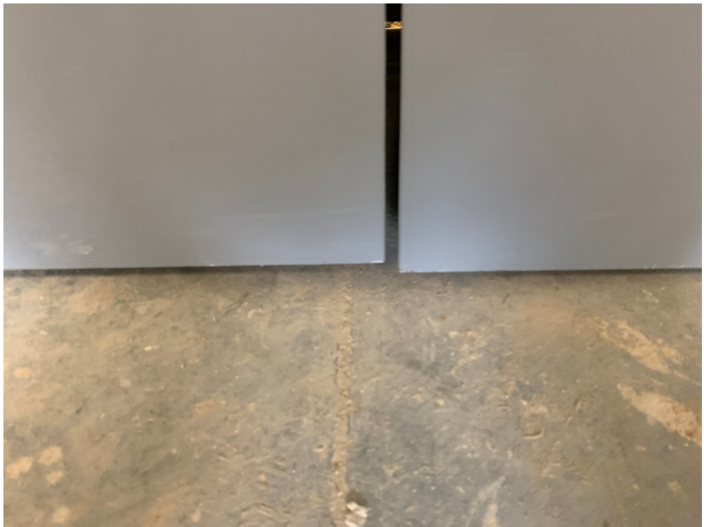
Figure 6 – Doors are out of Square at Entry Into new Addition
