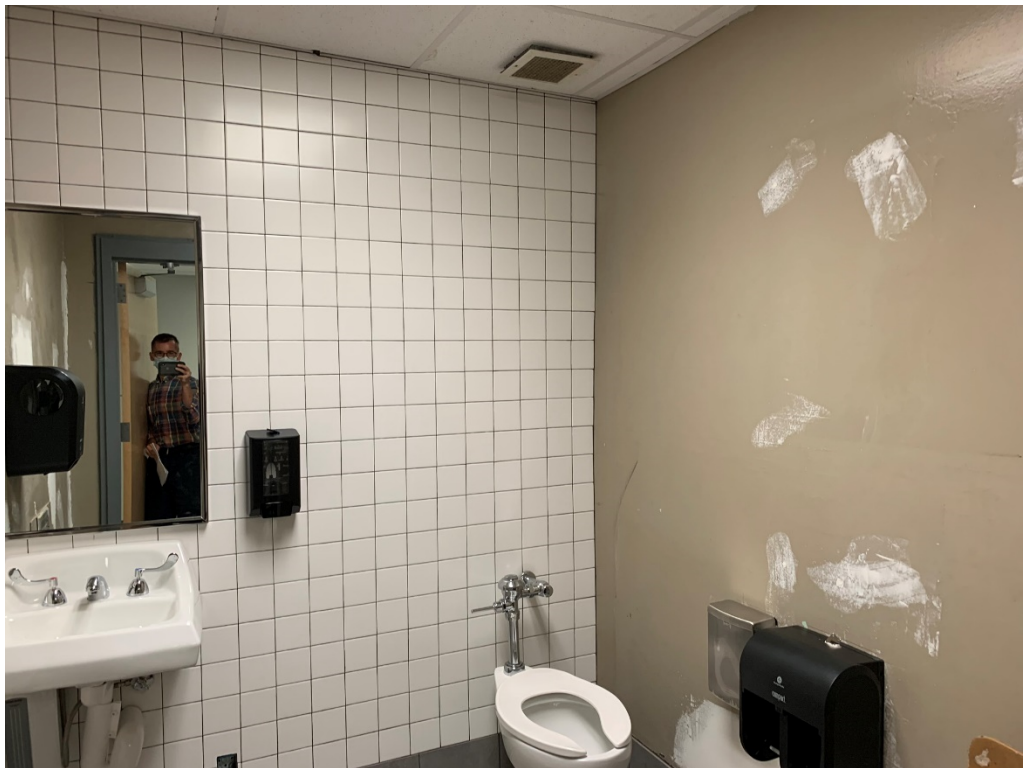
Figure 2 – Teacher Bathroom in South Hall
