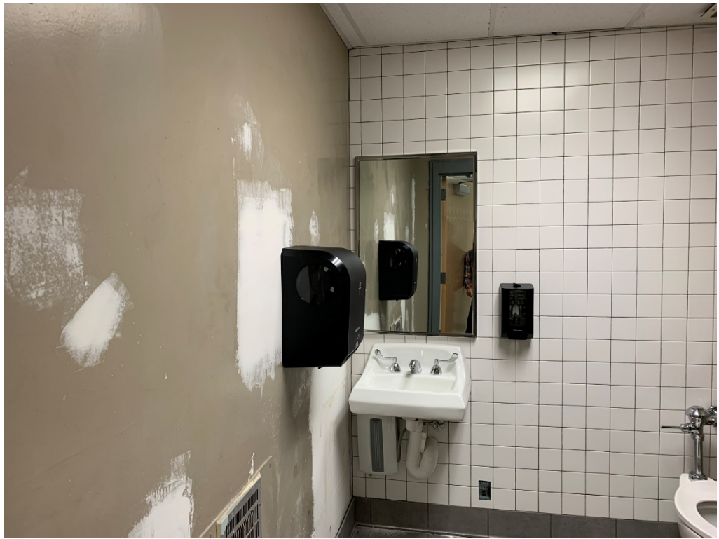
Figure 1 – Teacher Bathroom in South Hall
