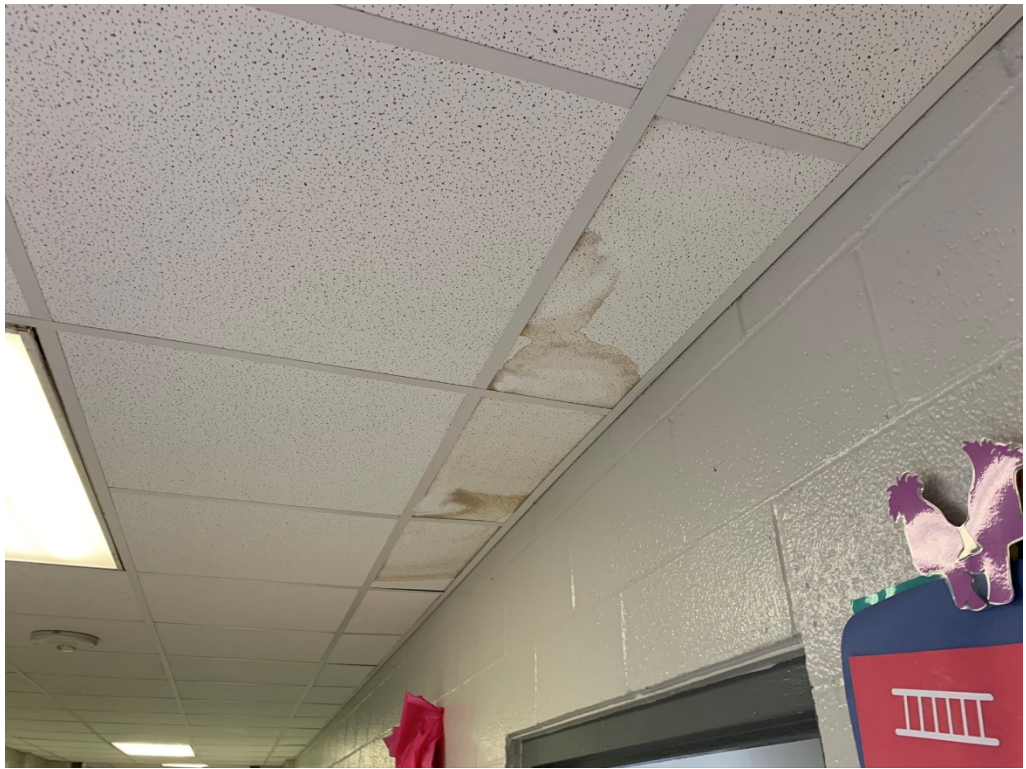
Figure 5 – A New Leak at ceiling Tile Near Class Near Auditorium
