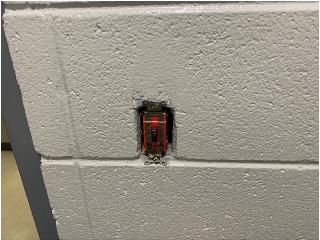
Figure 7 – Several Electrical Code Violations need to be Remedied ASAP
