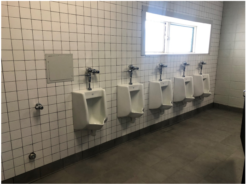
Figure 13 – Missing Urinal Installed
