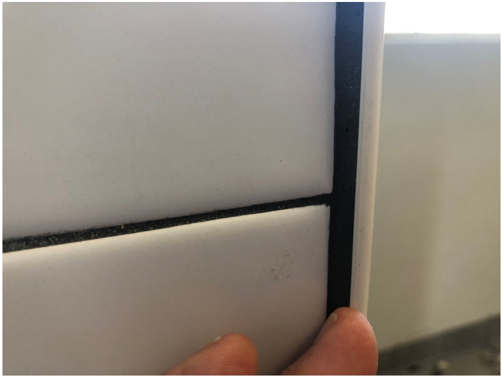
Figure 15 – Edge Trim Protrudes 1/8" +/-
