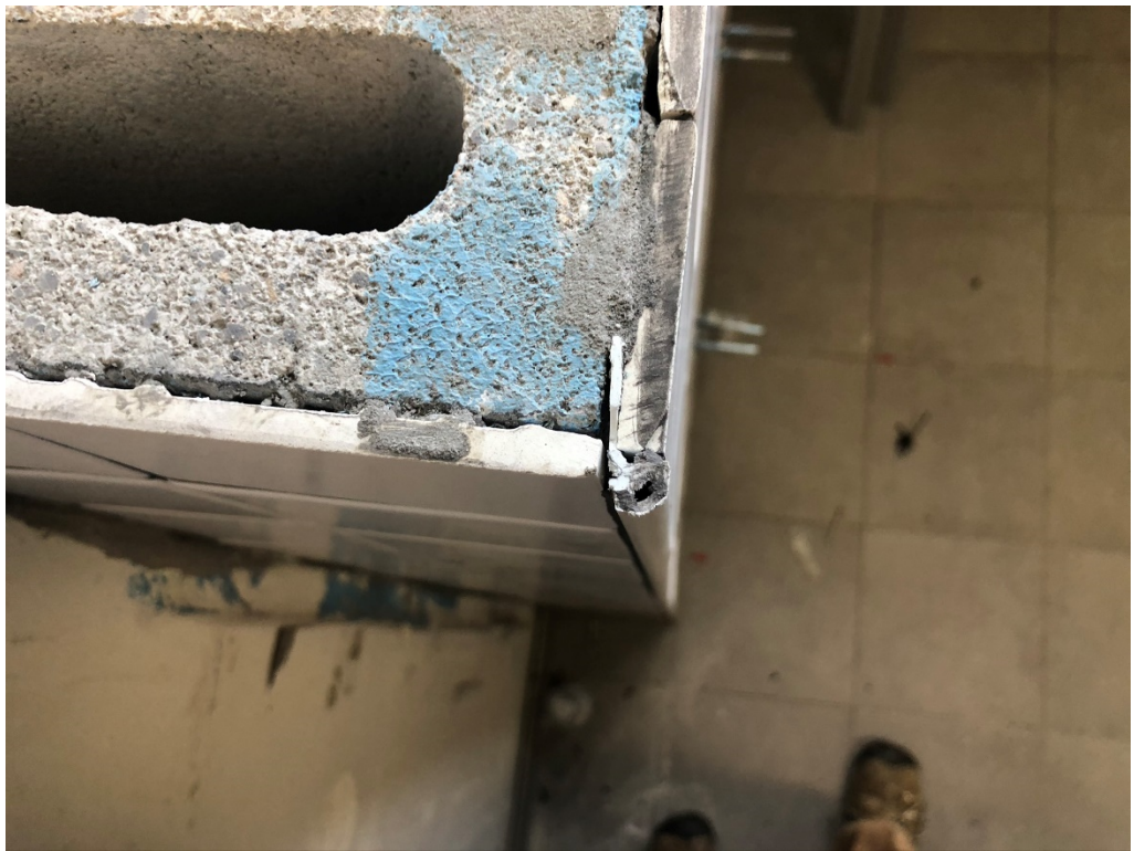
Figure 16 – Edge Trim Protrudes 1/8" +/-
