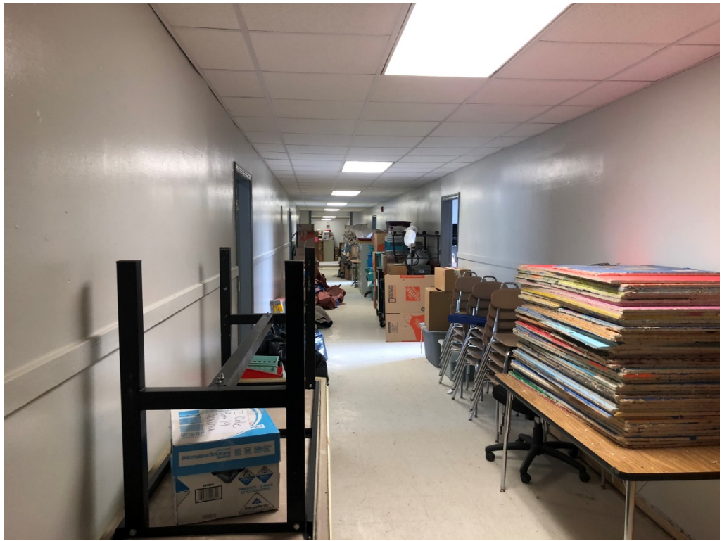
Figure 3 – After Contractor cleared hall, teachers moved items back into hall when swapping rooms; This could impede progress soon if not cleared for VCT install at Hallway
