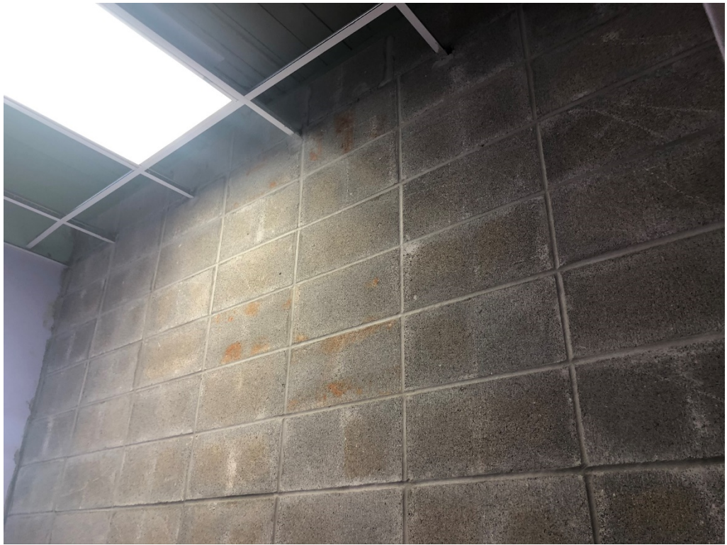
Figure 9 – Block Work at Girls T9 (Ceiling Grid will Require edge Support at Ceiling/Wall)
