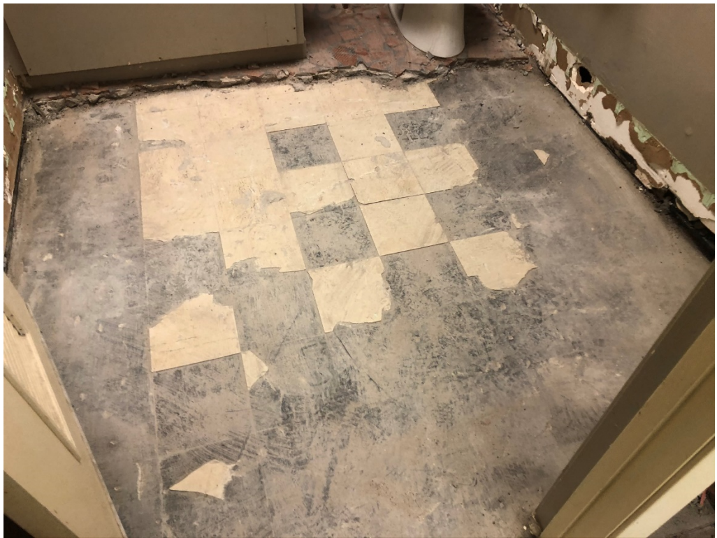
Figure 2 – Demo @ Staff Bathroom T7
