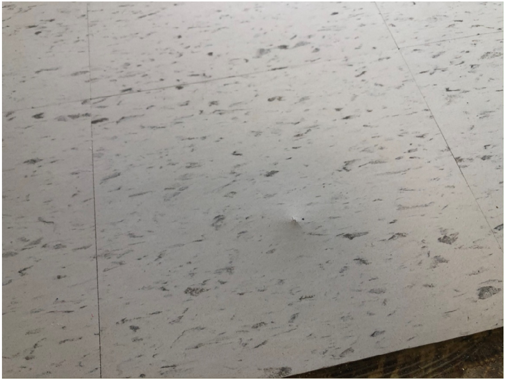
Figure 13 – Some Damage Noted at VCT at Entry to Classroom 5
