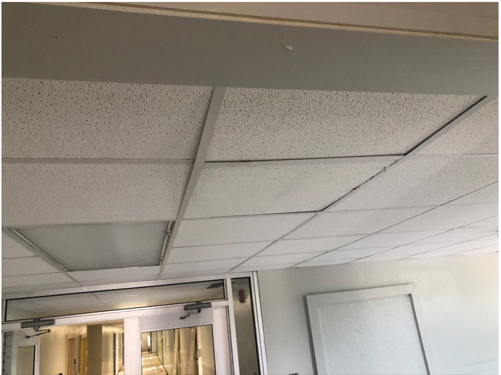
Figure 14 – Damage to Ceilings Noted after School Technical Staff Site Visit
