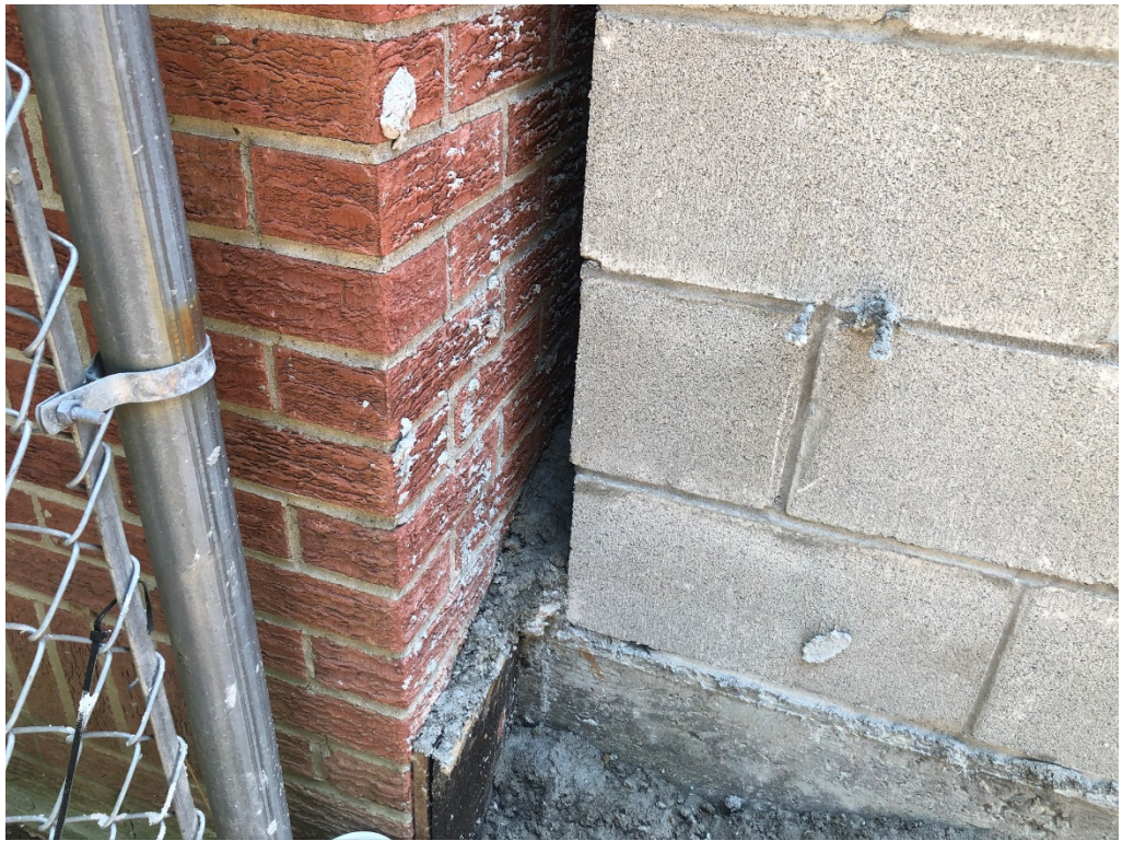
Figure 3 – Expansion joint Connection
