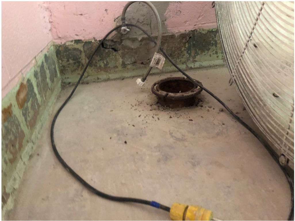
Figure 5 – Previous Large Mortar Bed in Bathrooms Requires Plumbing Rework for New
