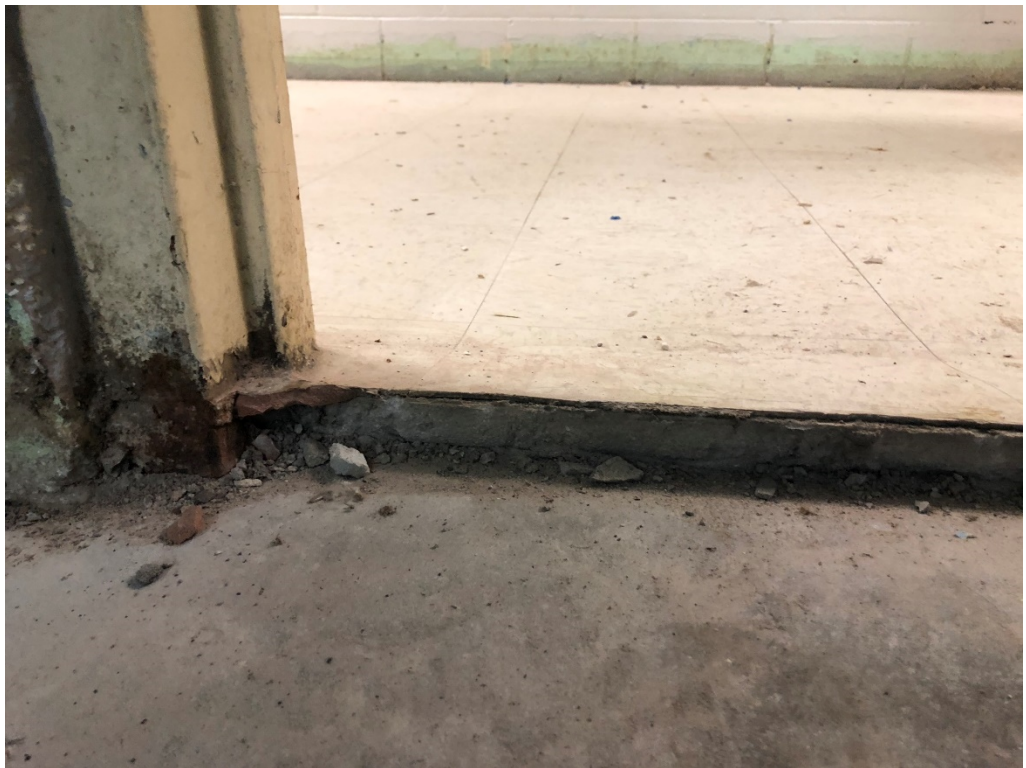
Figure 6 – Previous Large Mortar Bed in Bathrooms Requires Threshold Rework for New
