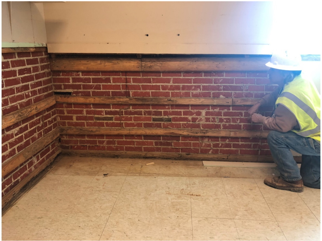
Figure 7 – Note Shims Under Base CC ~36"
