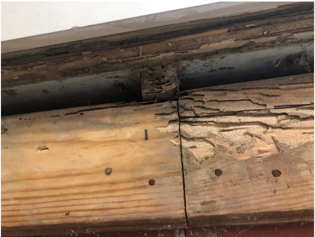
Figure 6 – Termite Damage @ Base Plate
