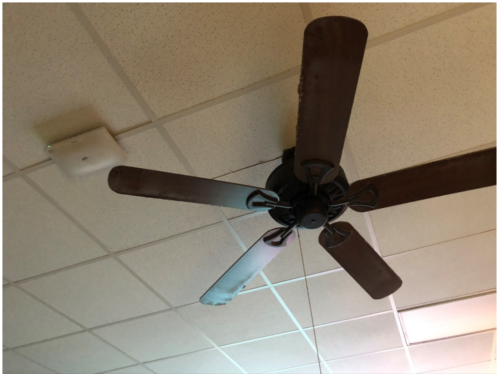
Figure 6 – Some Ceiling Tile Edges Unsupported
