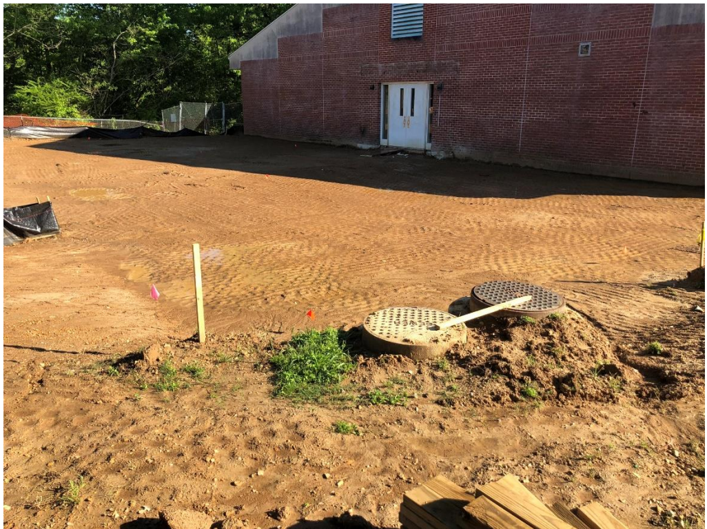
Figure 4 – Building pad Appears at grade
