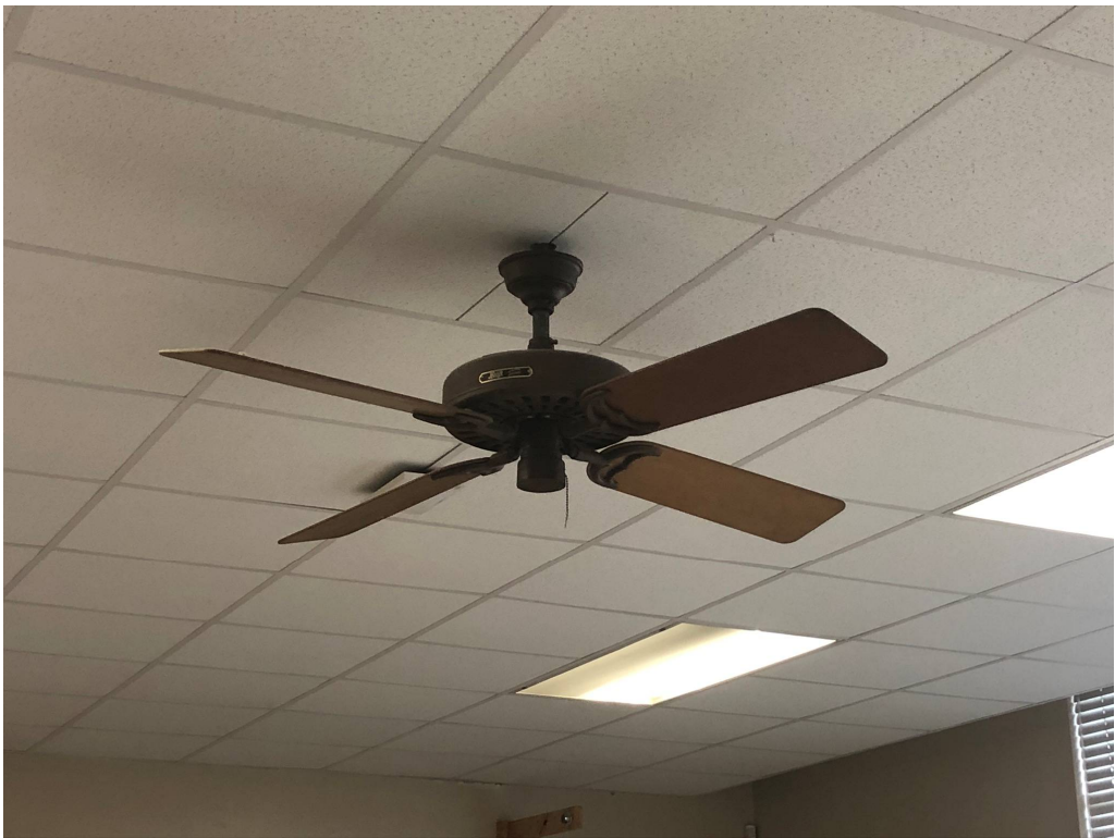
Figure 4 – Some Classrooms @ Ceiling Fans still Need Grid Completed
