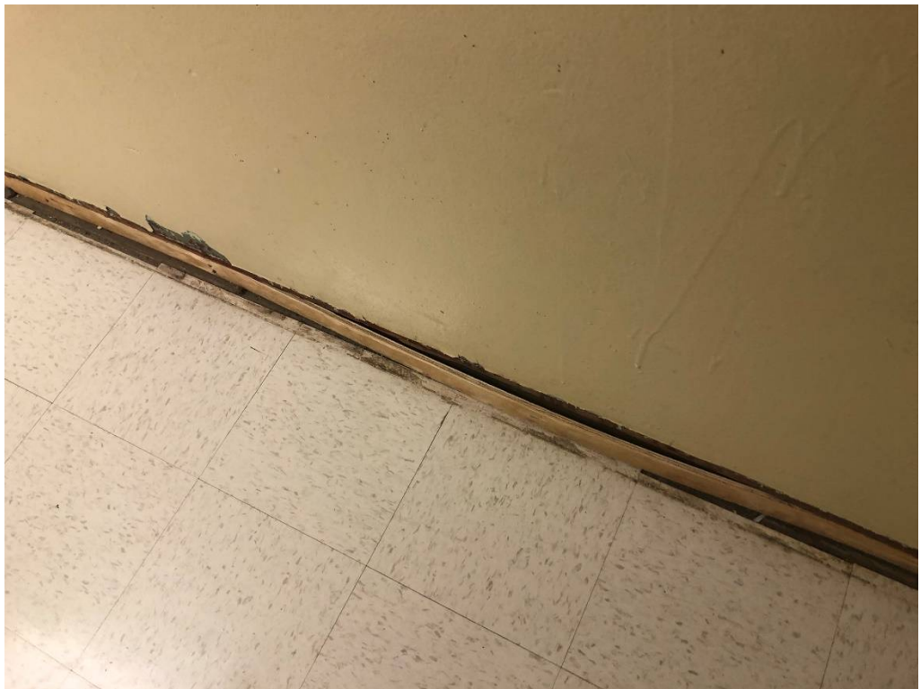
Figure 22 – Bulge in Plywood will prevent Base from Laying Flat
