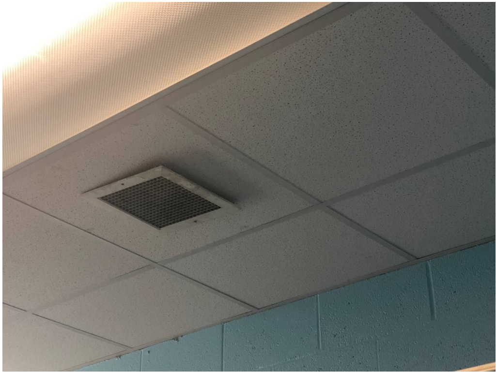
Figure 13 – Hanging Vent at Ceiling in Boys T5
