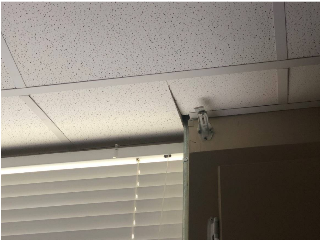
Figure 12 – Unfinished Corner @ Nurse Room 26
