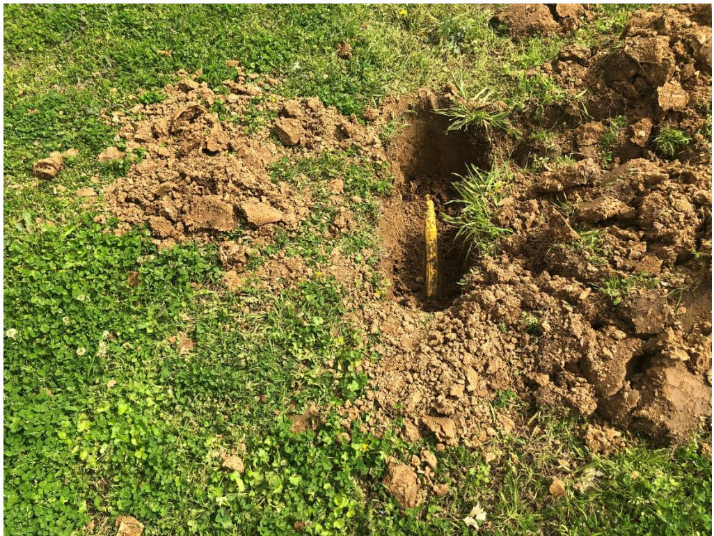
Figure 2 – Gas Pipe Uncovered Between Halls at Exterior
