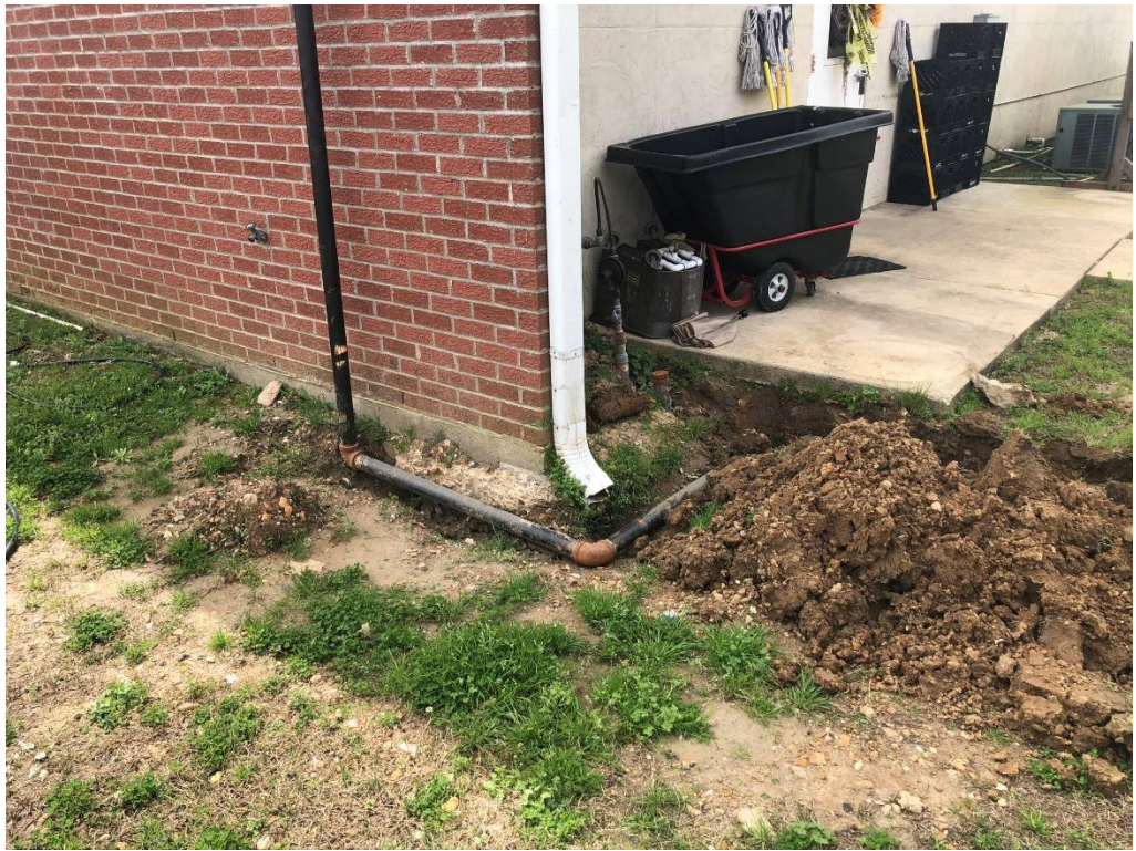
Figure 1 – Gas Line Uncovered at NW Corner of South Hall/Cafeteria
