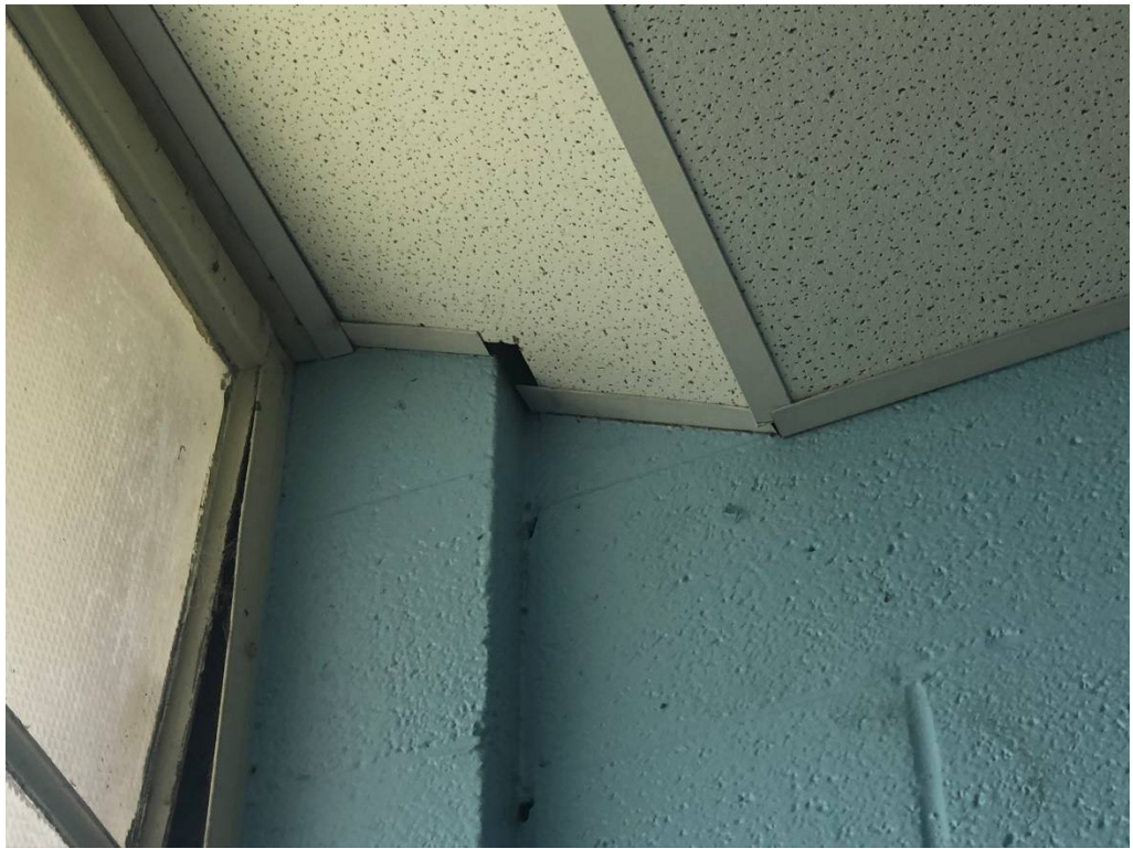
Figure 15 – Unfinished Corner at Ceiling in Boys T5
