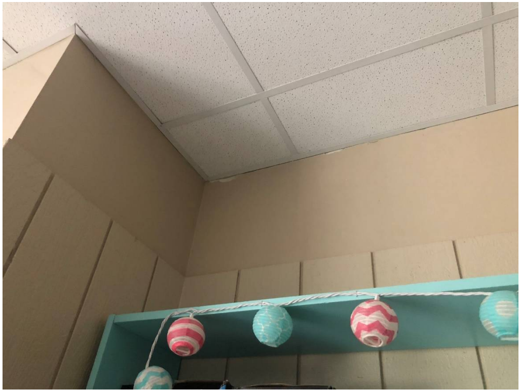
Figure 7 – Some Wall Damage Noted in Classroom 14 on North Hall
