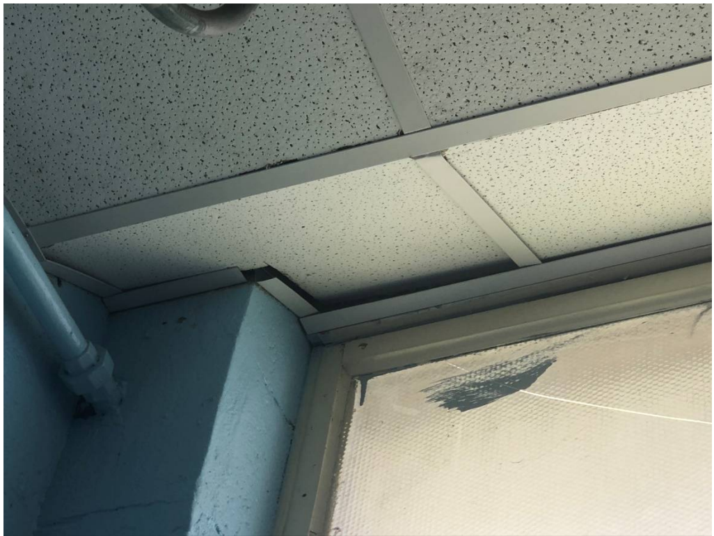
Figure 14 – Unfinished and Offset Corner at Ceiling in Boys T5
