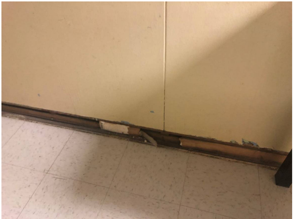
Figure 6 – Lower Section of Drywall Requires Smooth/Solid Backing for Rubber Base Install
