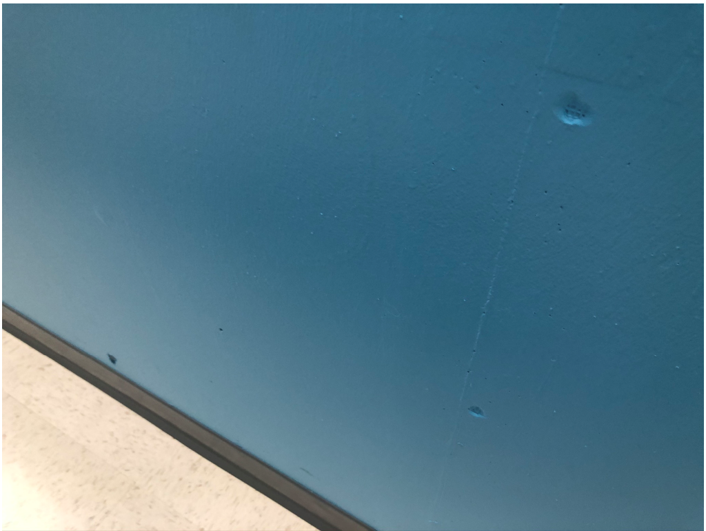
Figure 2 – Divots that should be Filled as is standard wall prep for paint
