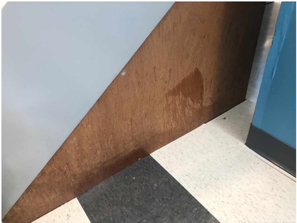
Figure 4 – Wax on Wall Panel & Missing Rubber Base
