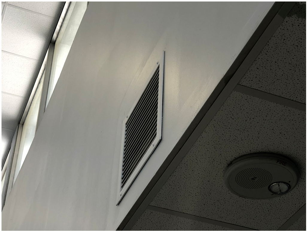
Figure 9 – Uneven Sheen at Walls in several Locations
