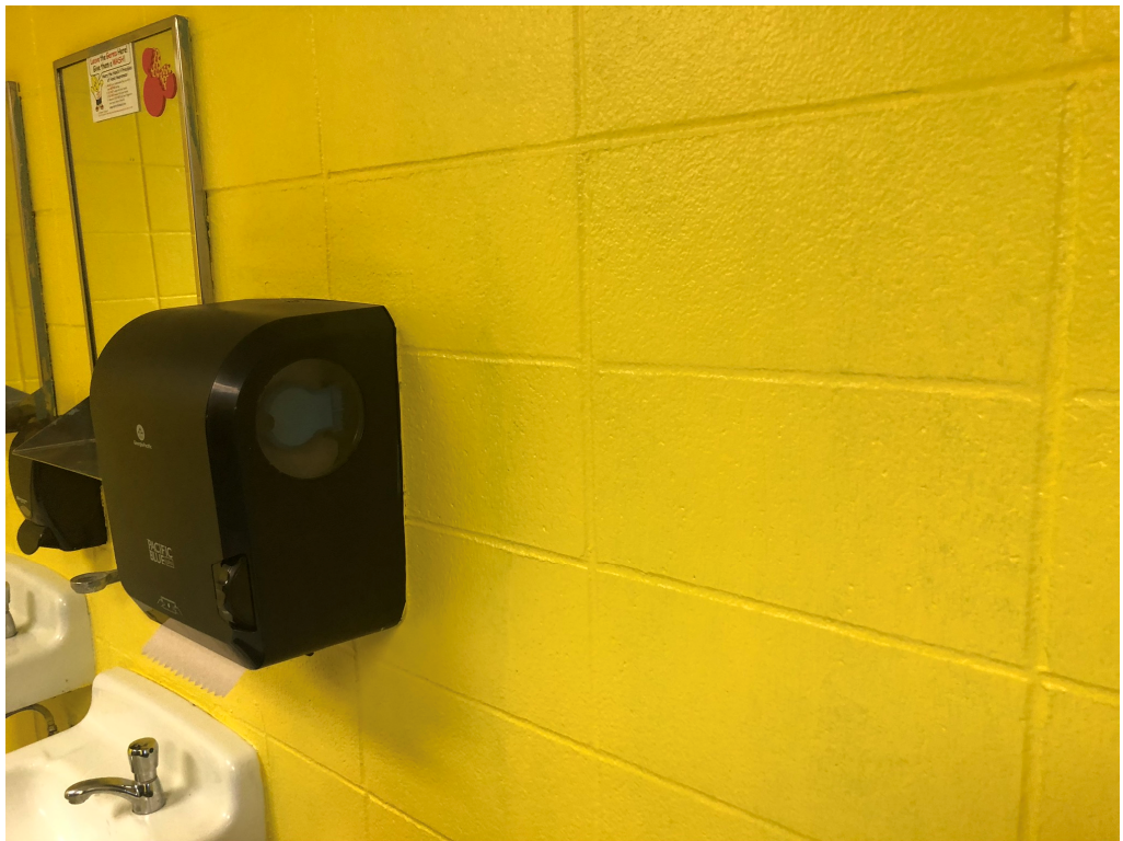
Figure 10 – Poor Paint Coverage
