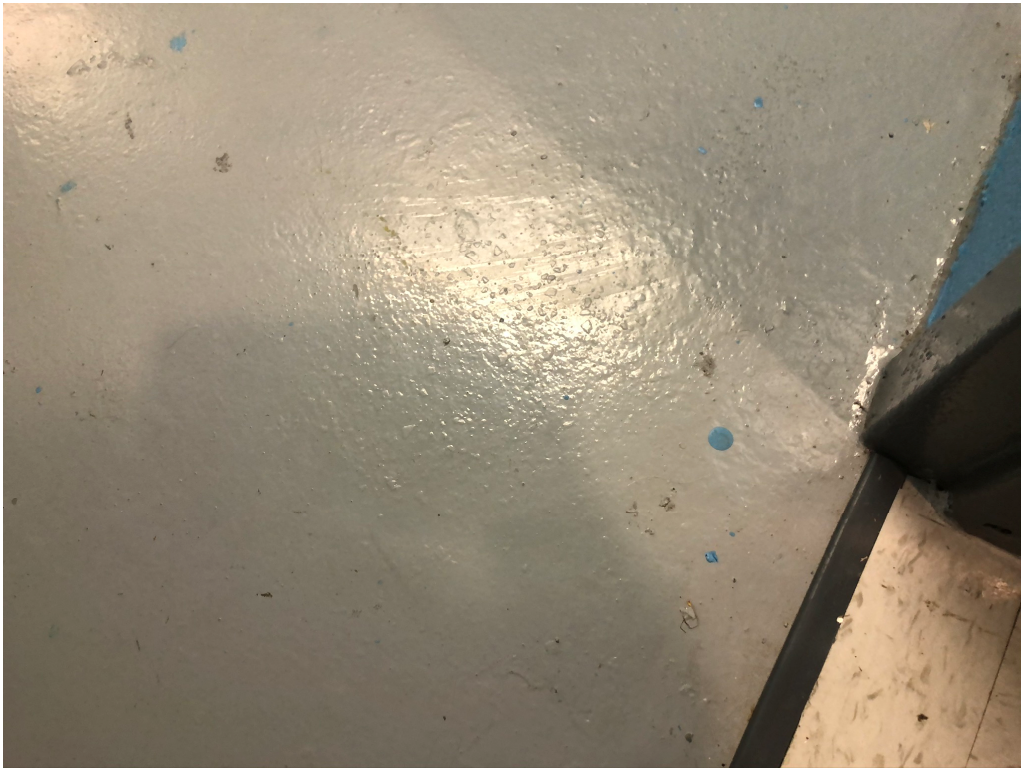
Figure 5 – Paint on Floors at Bathrooms
