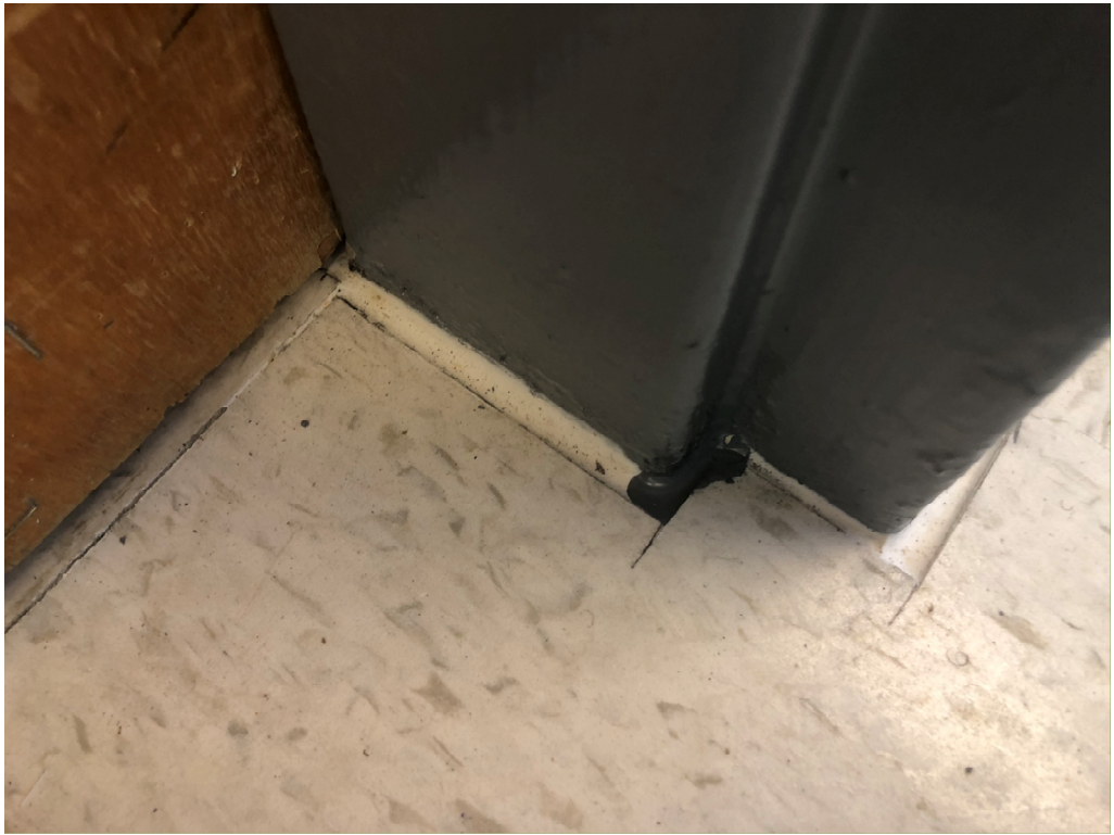
Figure 7 – Pencil Marks at Door Thresholds & Paint On Floor
