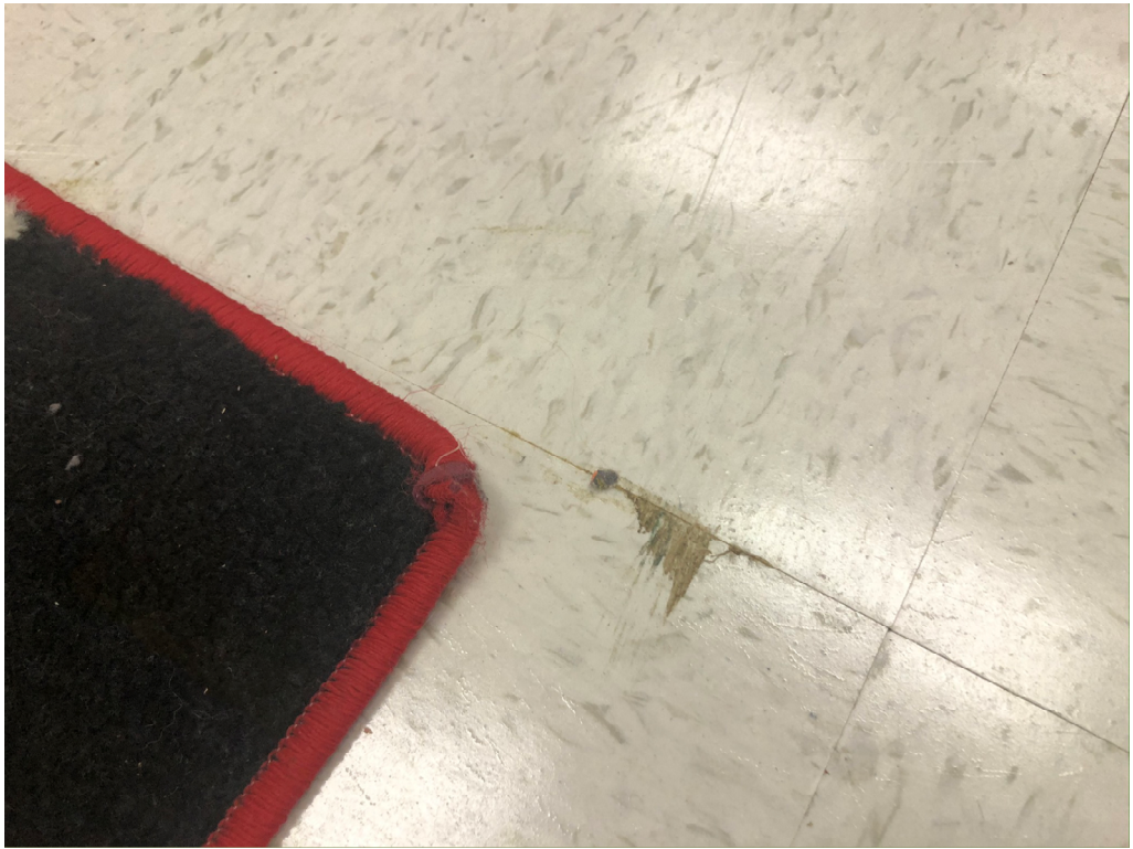
Figure 19 Glue at Floor Tiles
