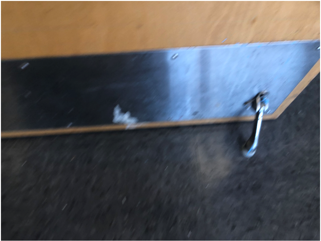
Figure 1 – Paint on Door
