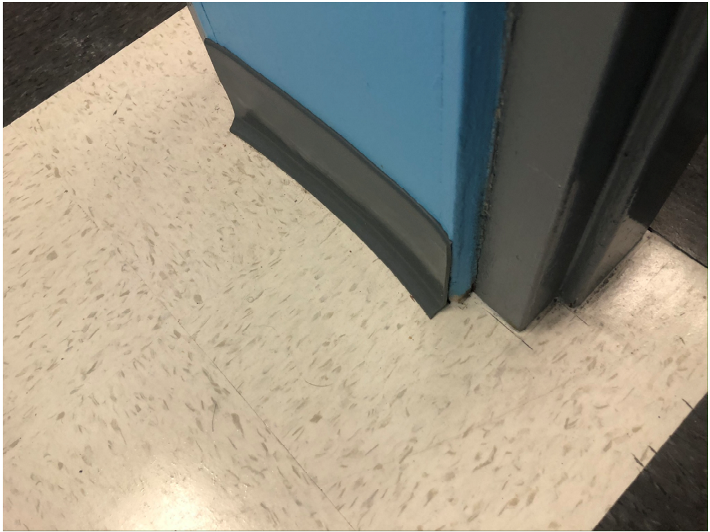
Figure 15 – Base Not Wrapped Around Corner
