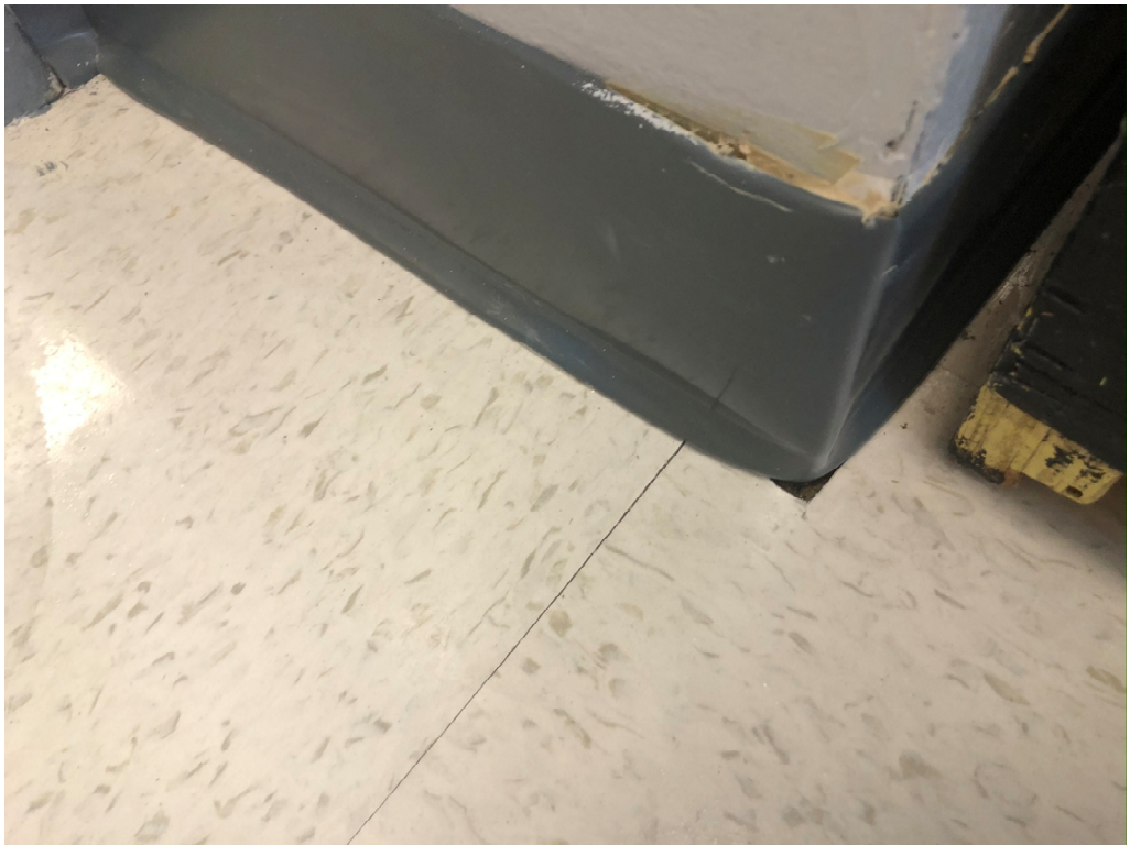
Figure 16 – Poorly Adhered Base and Unmitered/Preformed corners
