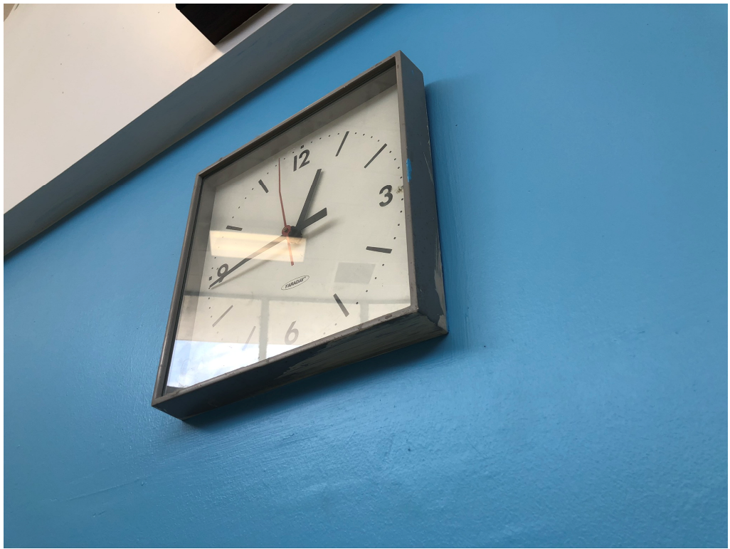
Figure 23 – Paint at School Owned Items
