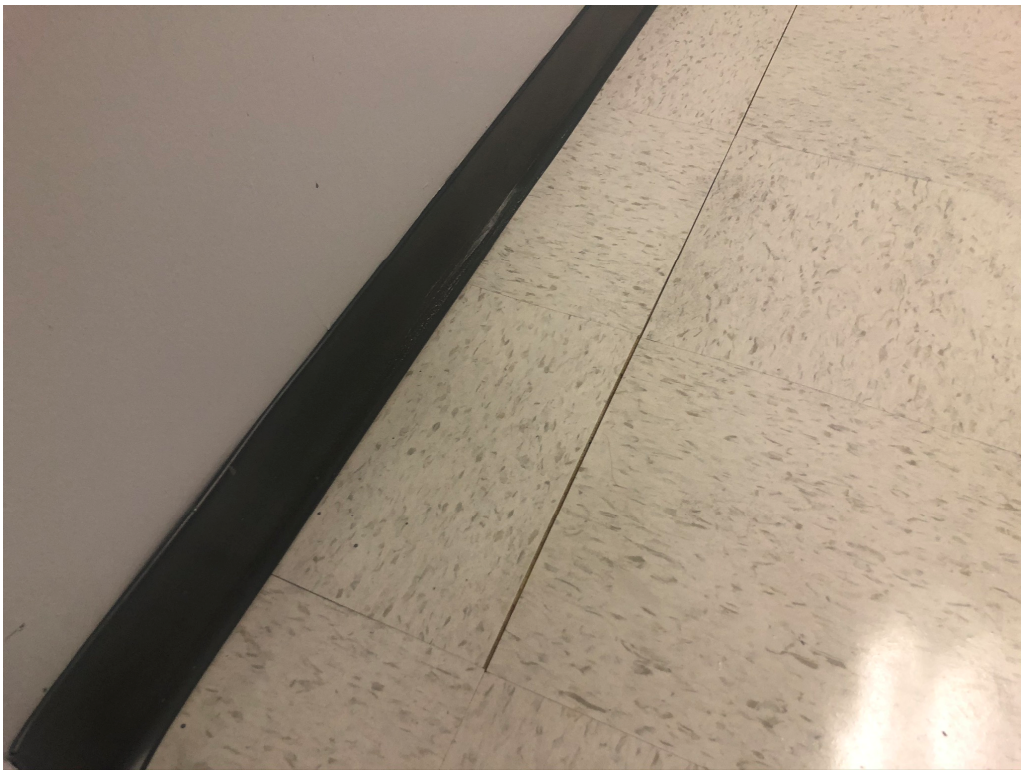
Figure 14 – Gaps Between Tiles
