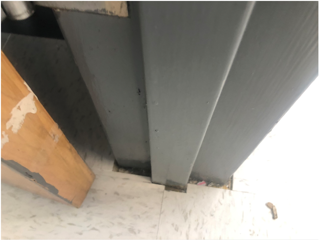
Figure 7 – Poorly notched Tile at Jamb
