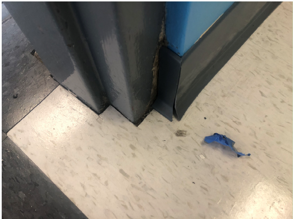
Figure 2 – Rubber Base Corner does not meet up
