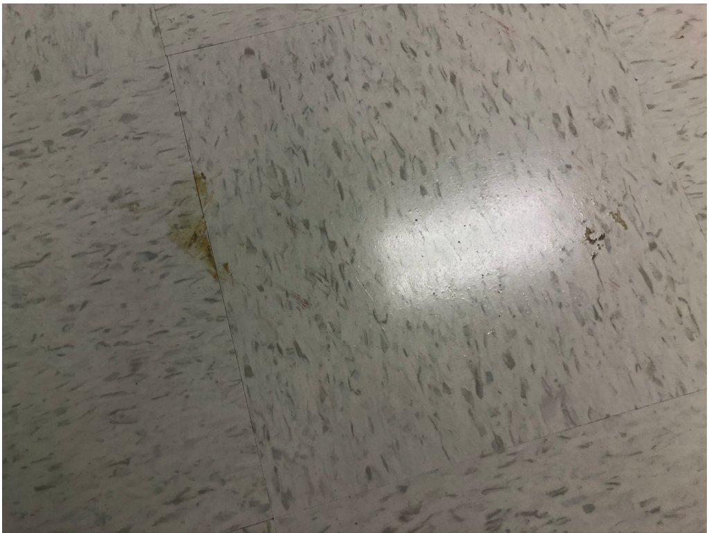
Figure 12 – Glue at Tile
