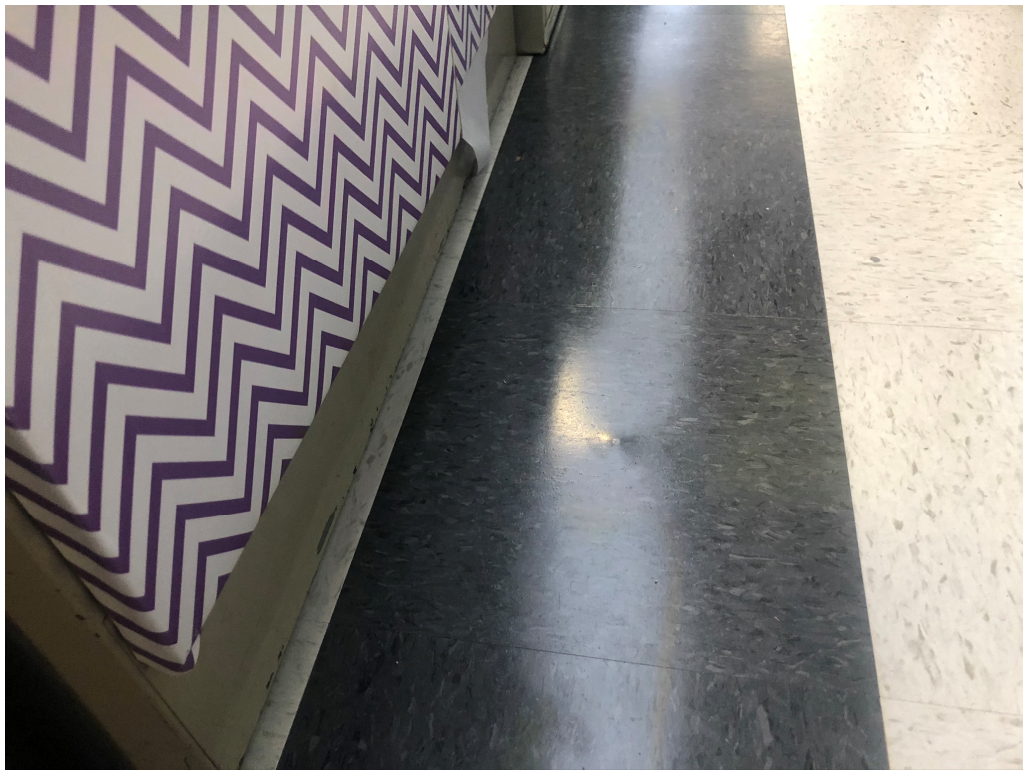
Figure 15 – Debris Under Tile
