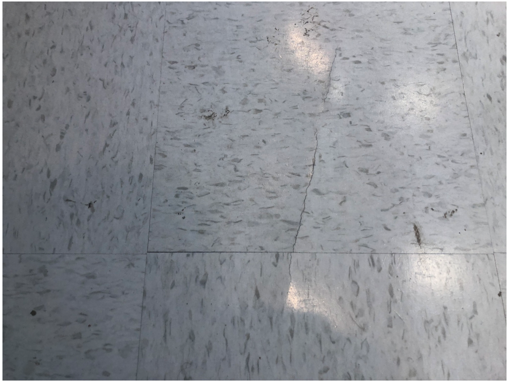
Figure 9 – Cracked Tile due to debris and/or lacked of floor prep
