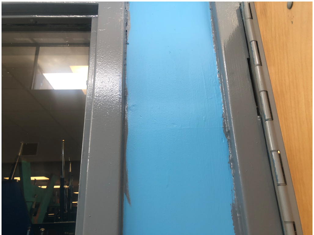
Figure 16 – Some Paint Touchups Required at Jambs and Walls
