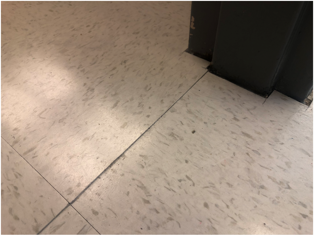
Figure 13 – Floor Tiles Mainly Around Thresholds and Floor Perimeters Not Flush
