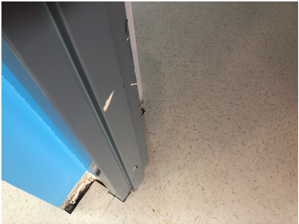
Figure 14 – Peeling Paint at Door Jambs
