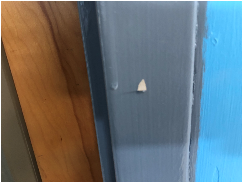
Figure 8 – Peeling Paint at Door Jambs
