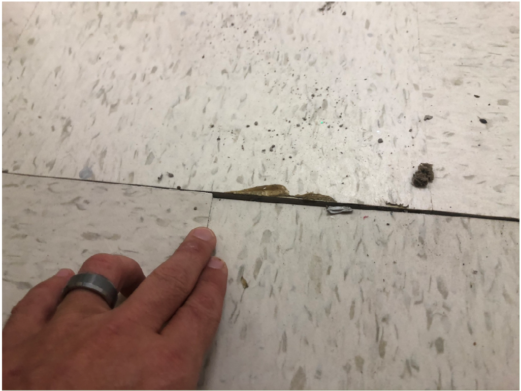
Figure 17 – VCT at Library Threshold is uneven and Needs to be reworked
