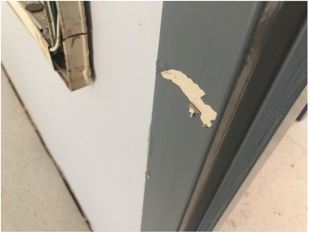
Figure 7 – Peeling Paint at Door Jambs
