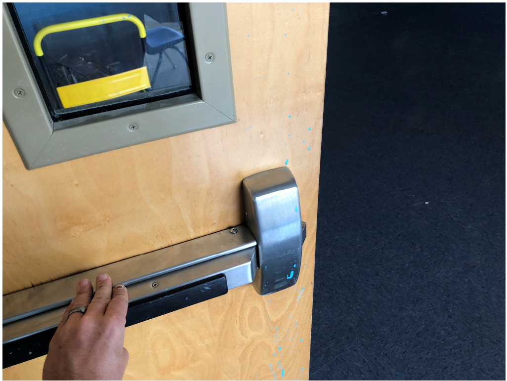
Figure 3 – Paint on Door Noted in Building 100
