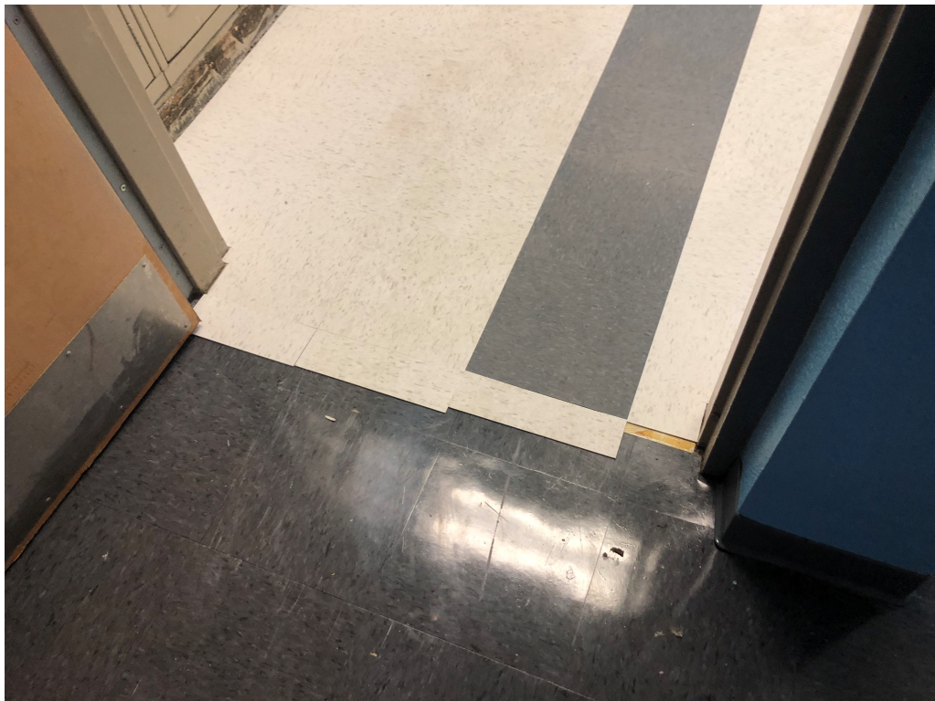
Figure 6 – Threshold @ Main Entrance Lobby and 300 Wing; These should meet Flush
