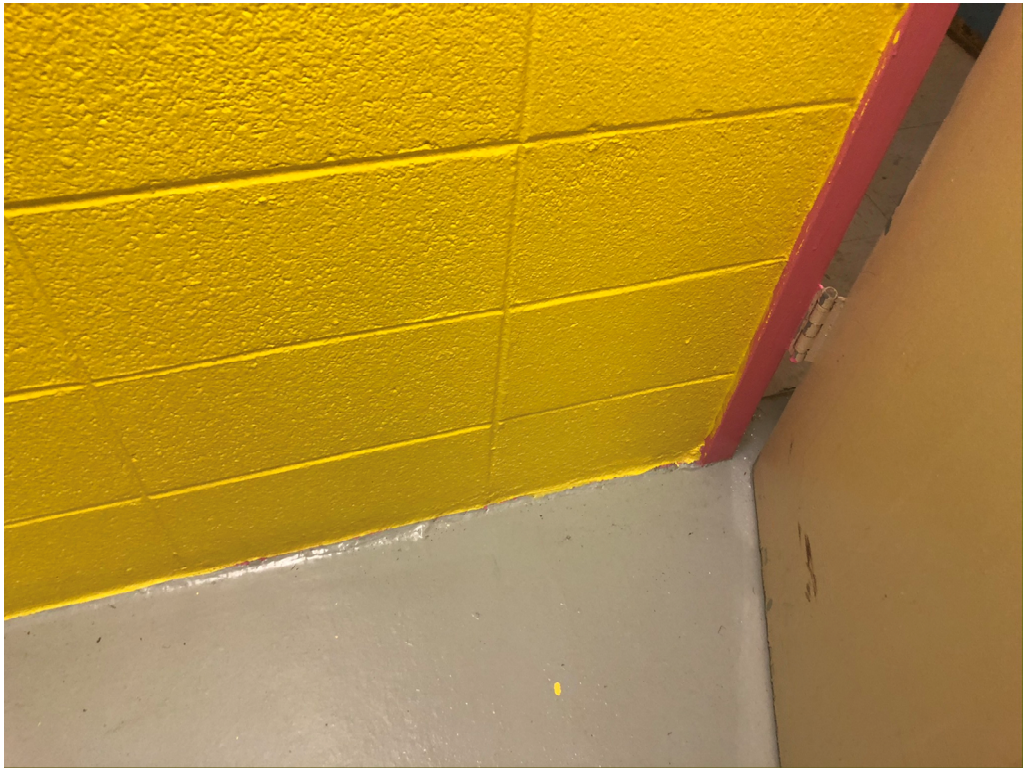
Figure 7 – This Line needs to be Straightened
