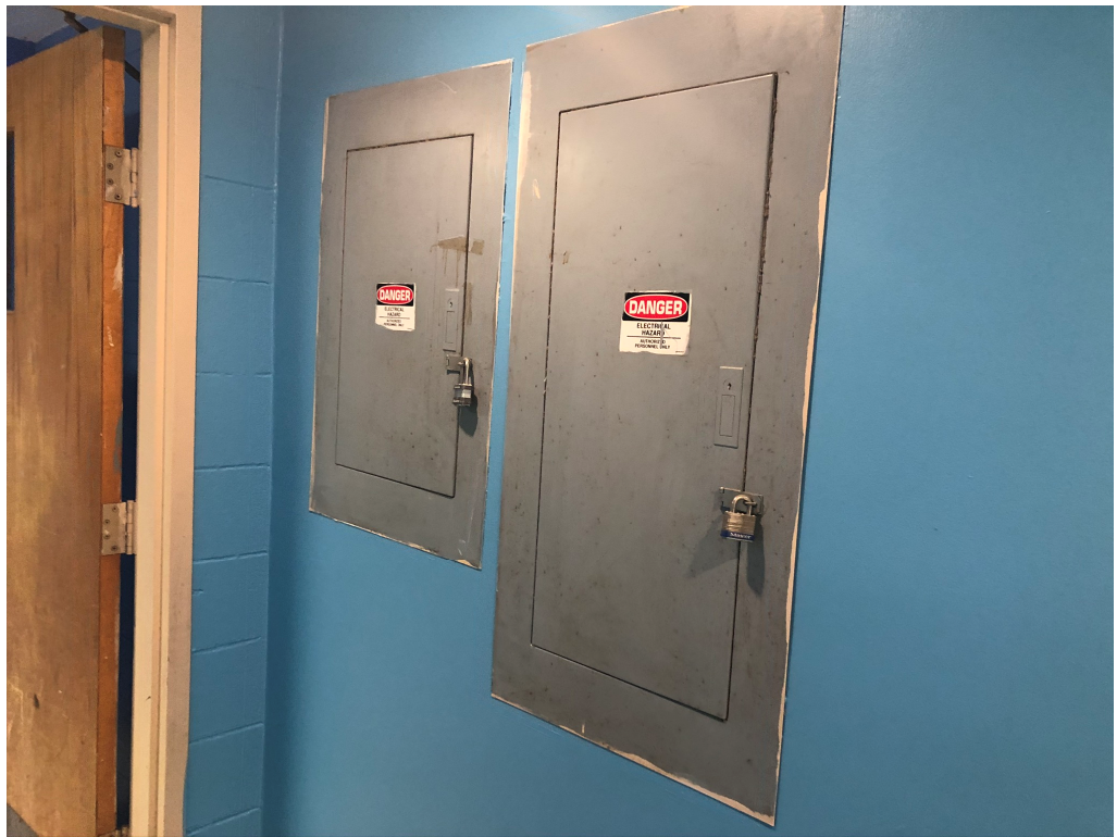
Figure 4 –Electrical Box Panels
