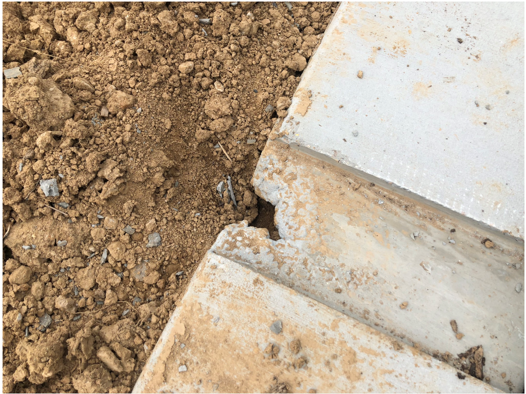
Figure 7 – Can we fill this recess with a Cementitious material and repair this void?
