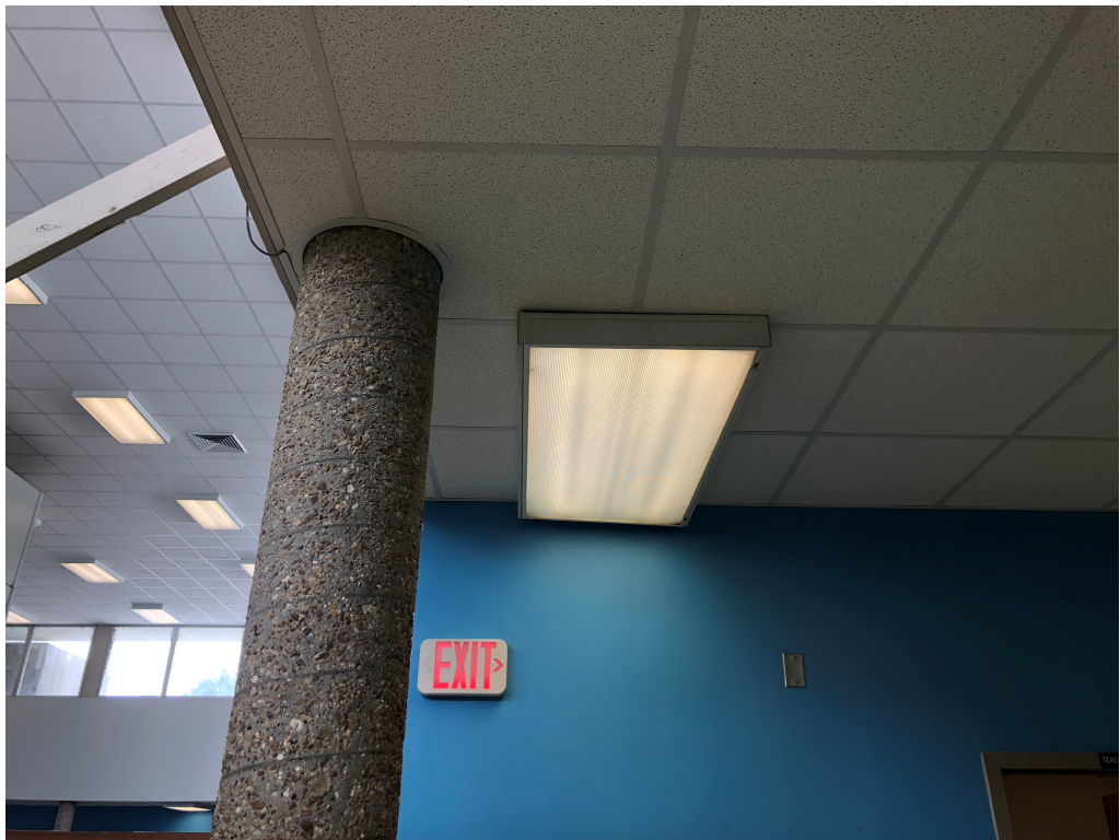
Figure 4 – This light in Building 3 has a gap on 2 corners and is not flush with ceiling
