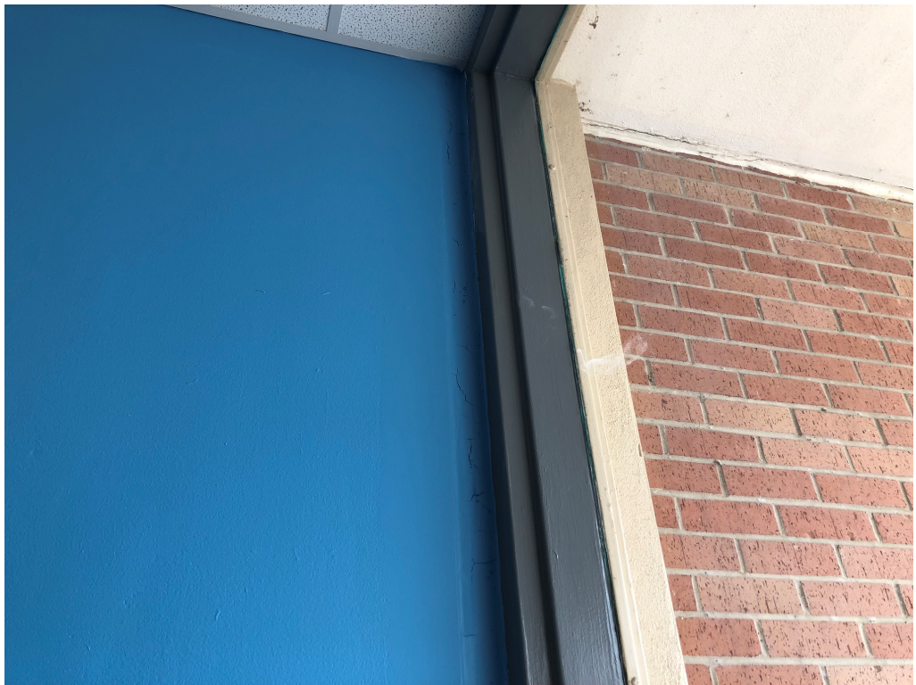
Figure 8 – The drywall at this window Jamb needs patching in Building 1 Lobby
