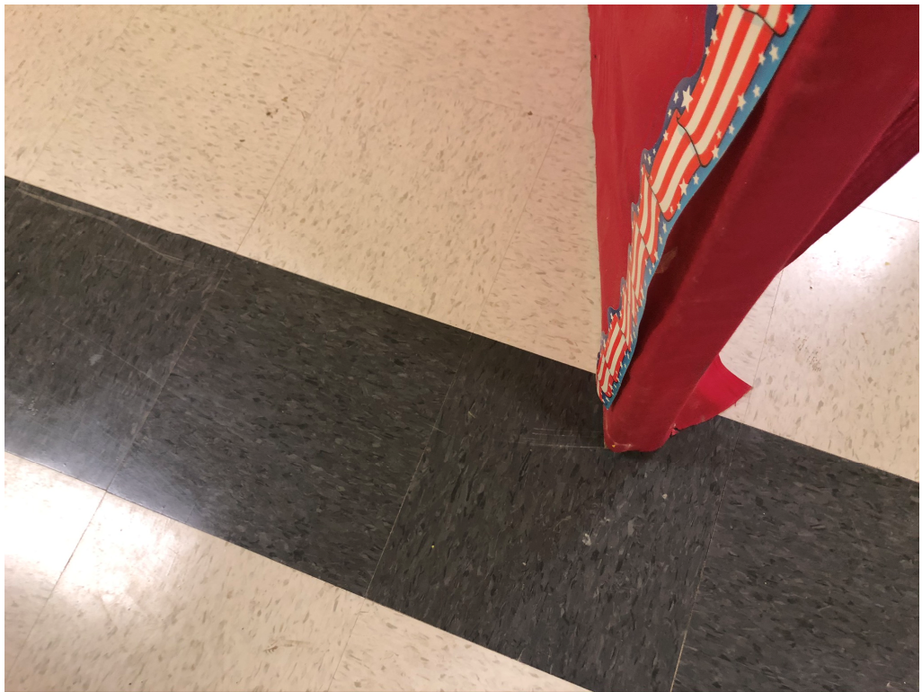
Figure 2 – Door dragging in hall needs undercut
