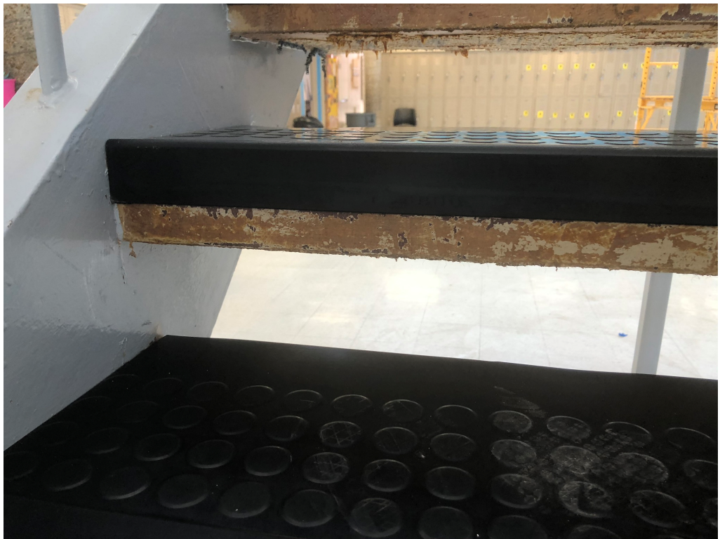
Figure 2 – Paint Required at lower section of tread as well as underneath and back side
