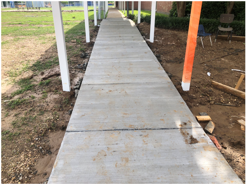
Figure 5 – Concrete Sidewalk Complete (dirt needs to be graded back to edge of walk)
