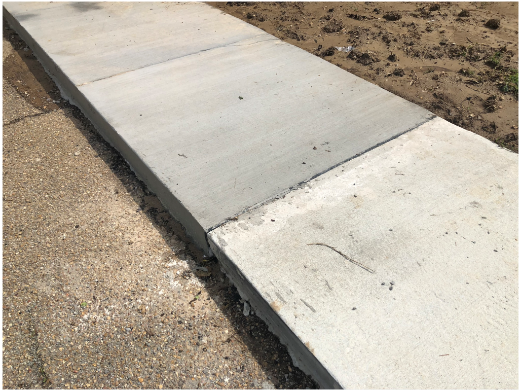
Figure 1 – Concrete Junction where new meets old
