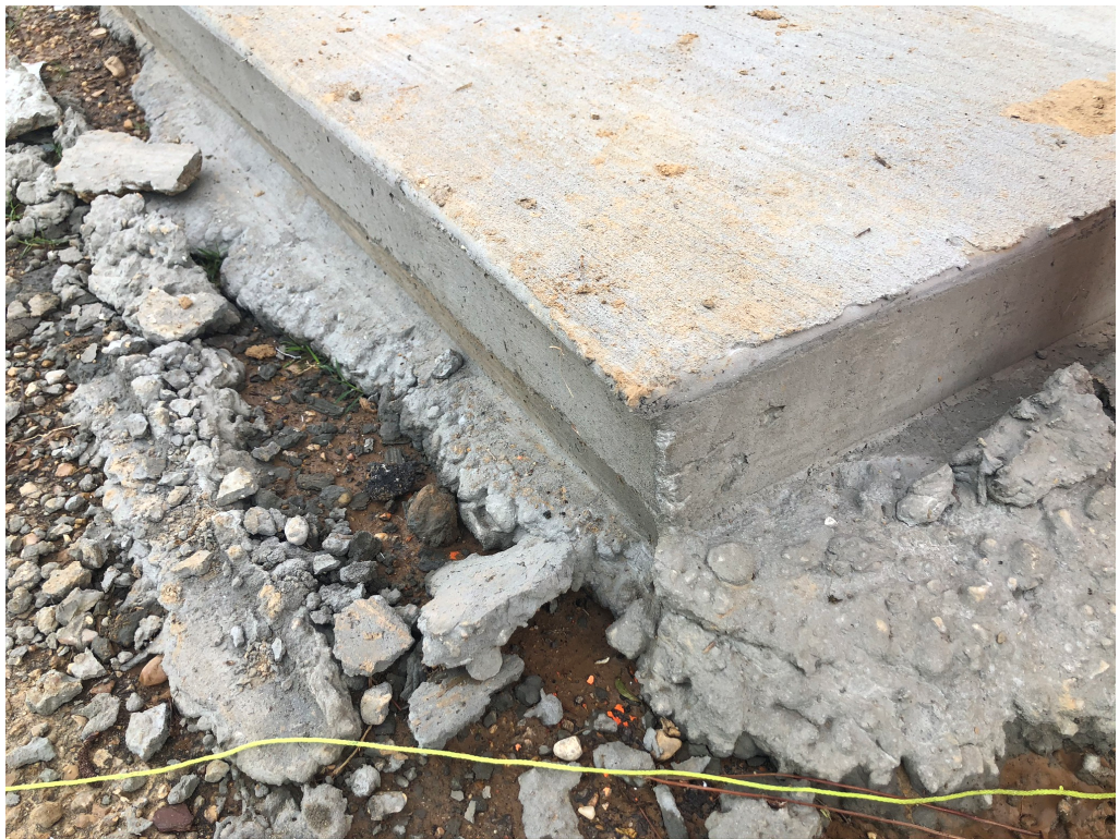
Figure 4 – Clean up edge of concrete that overhangs here (North Corner of Awning/walkway)
