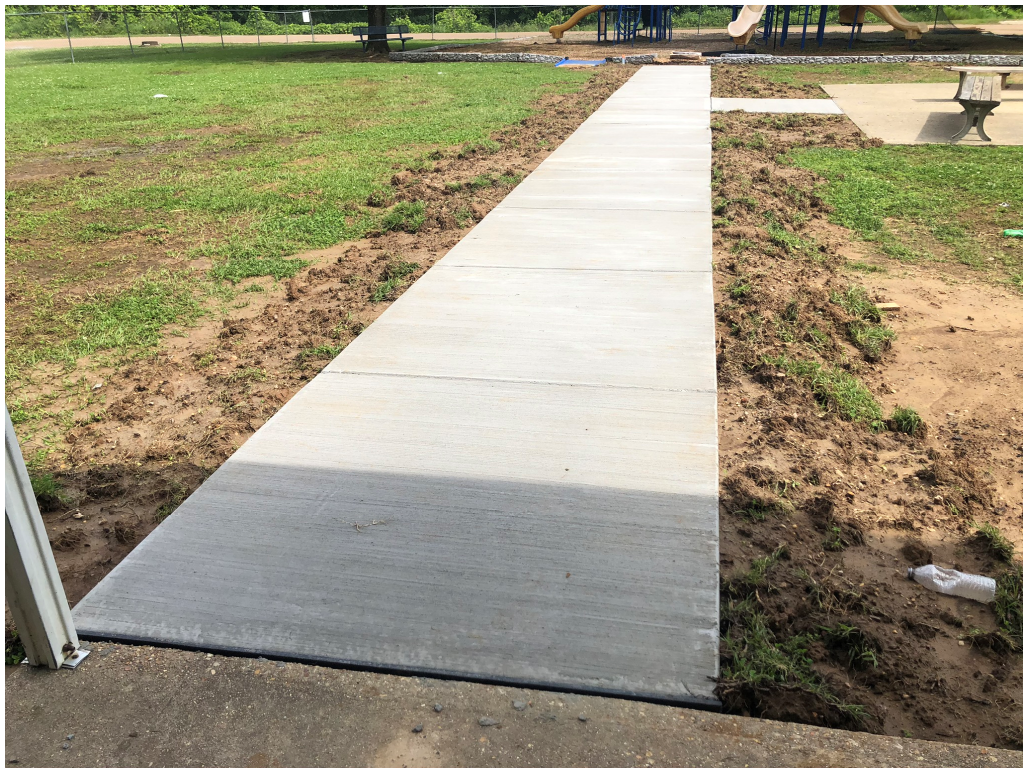
Figure 6 – Concrete Sidewalk Complete (dirt needs to be graded back to edge of walk)
