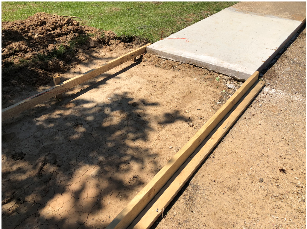
Figure 4 – Extent of Concrete
