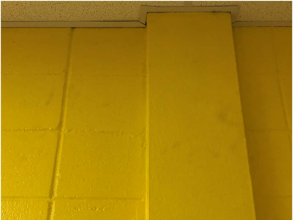
Figure 2 – Dirt Hand Marks (most likely from ceiling install)
