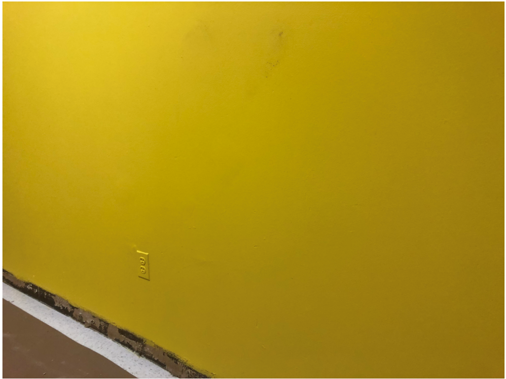
Figure 3 – Dirty Marks on Wall
