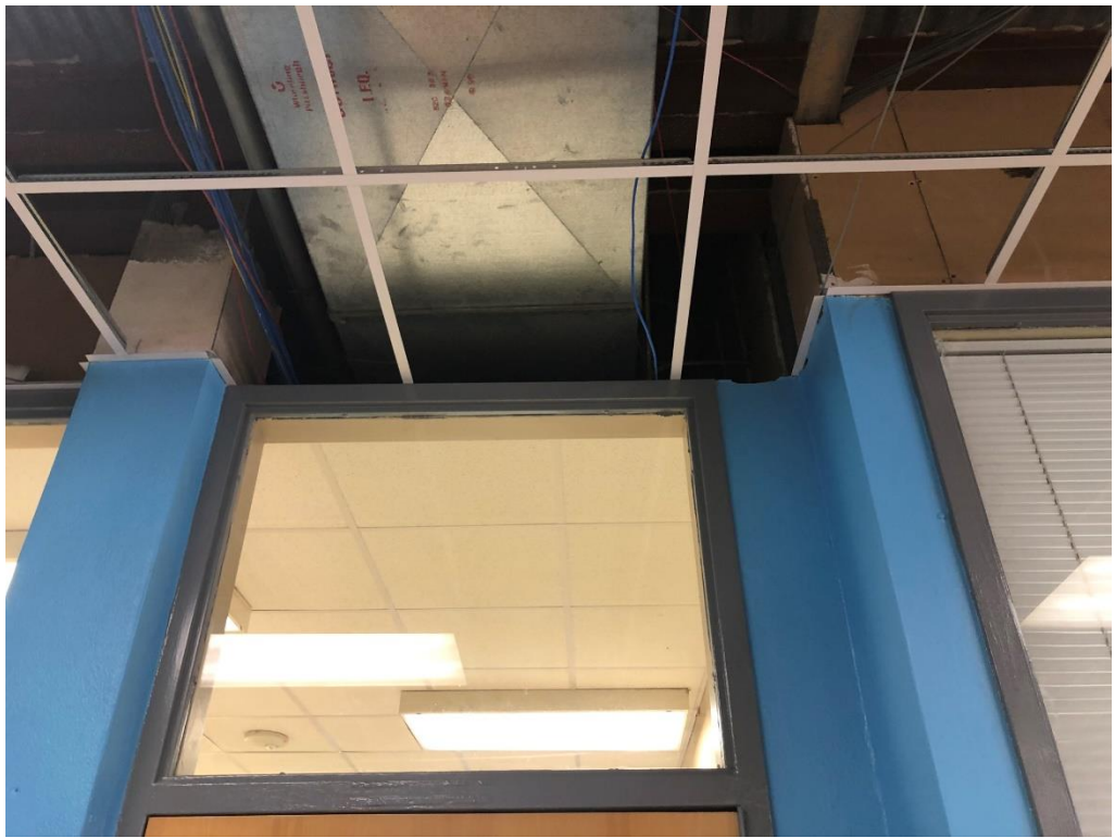
Figure 3 – Right of Door Frame Needs Corner Support
