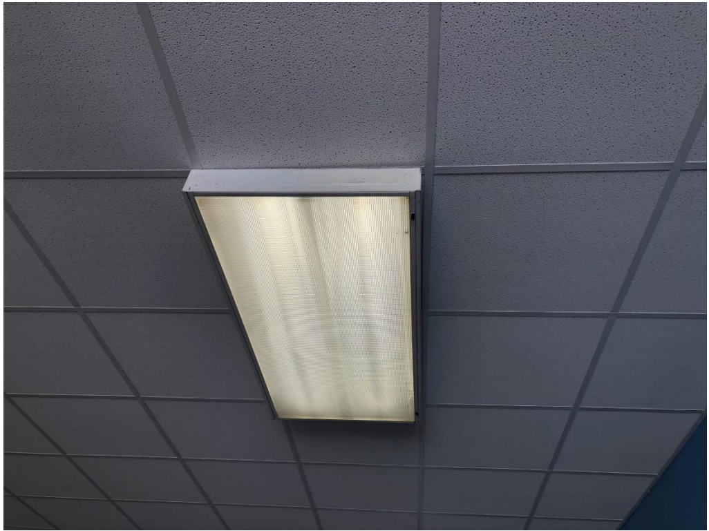
Figure 13 – Light Mis-aligned, Offset from Grid Center
