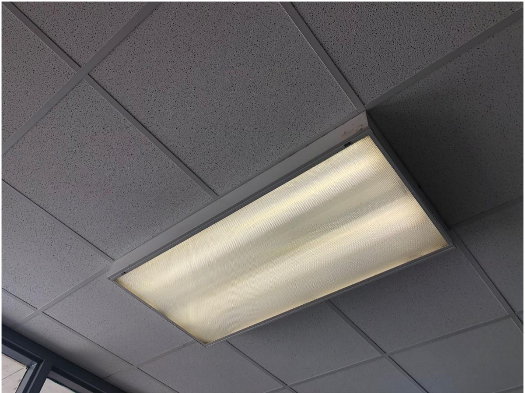
Figure 12 – Some Lights Not Lined up (at slight angle, needs correction)
