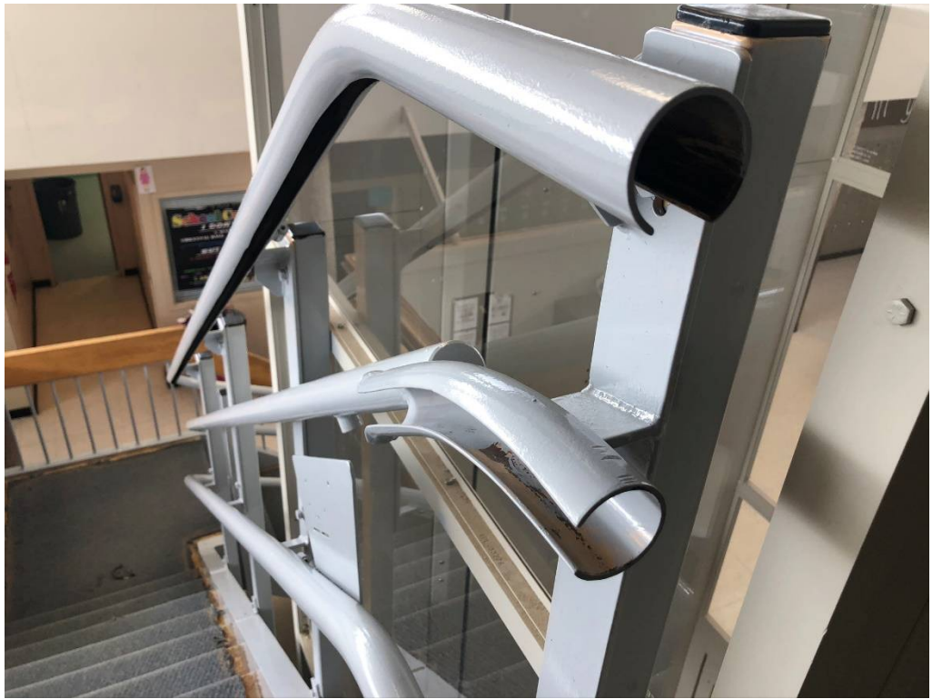
Figure 11 – South Stair in Building 3: Paint needed on visible bottom side of inner tube here
