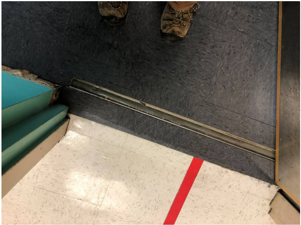
Figure 7 – Lobby B Threshold and Expansion Joint Covers Still Needed
