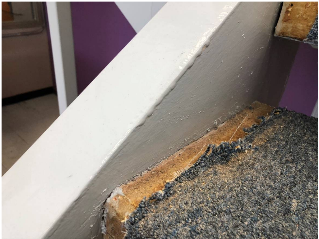
Figure 10 – South Stair in Building 3 has some paint buildup that requires sanding and refinishing
