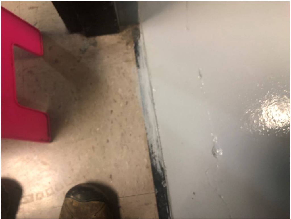
Figure 13 – Paint on Threshold in T06
