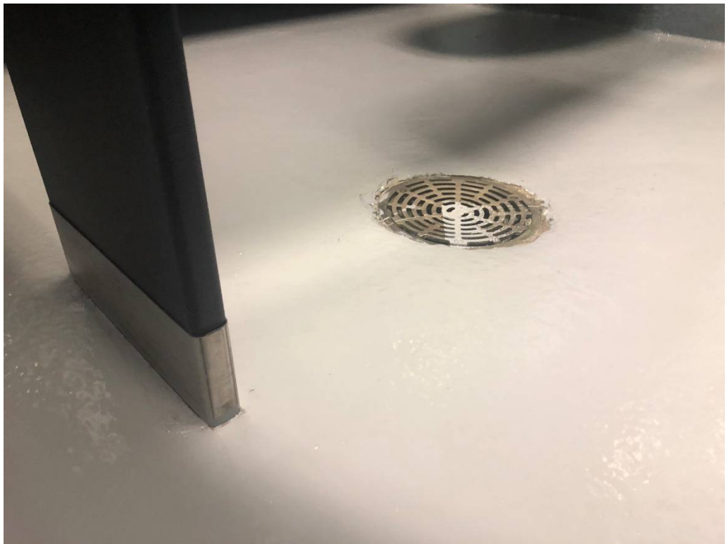
Figure 12 – Paint on Drain Cover in T06
