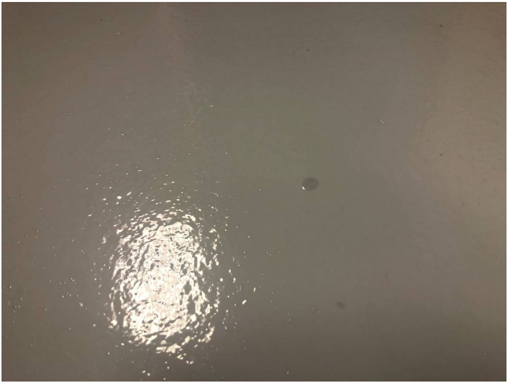
Figure 5 – Building 2 Gym (T06): discolored drips evident after install
