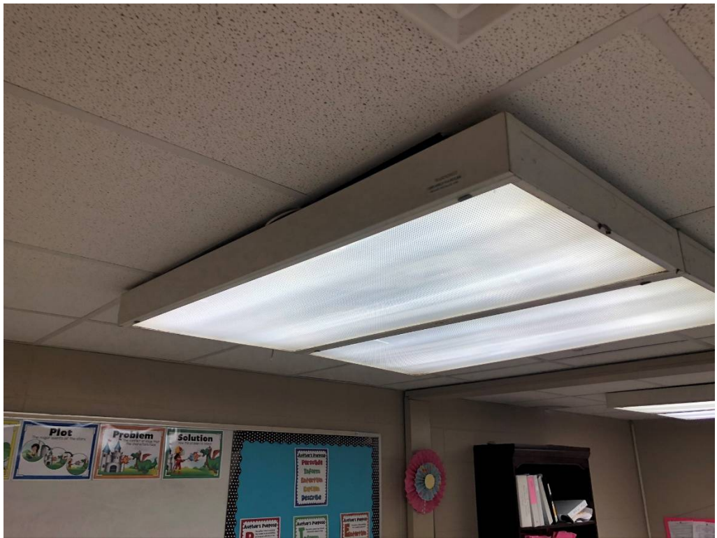
Figure 2 – Light Needs Adjusting in 304
