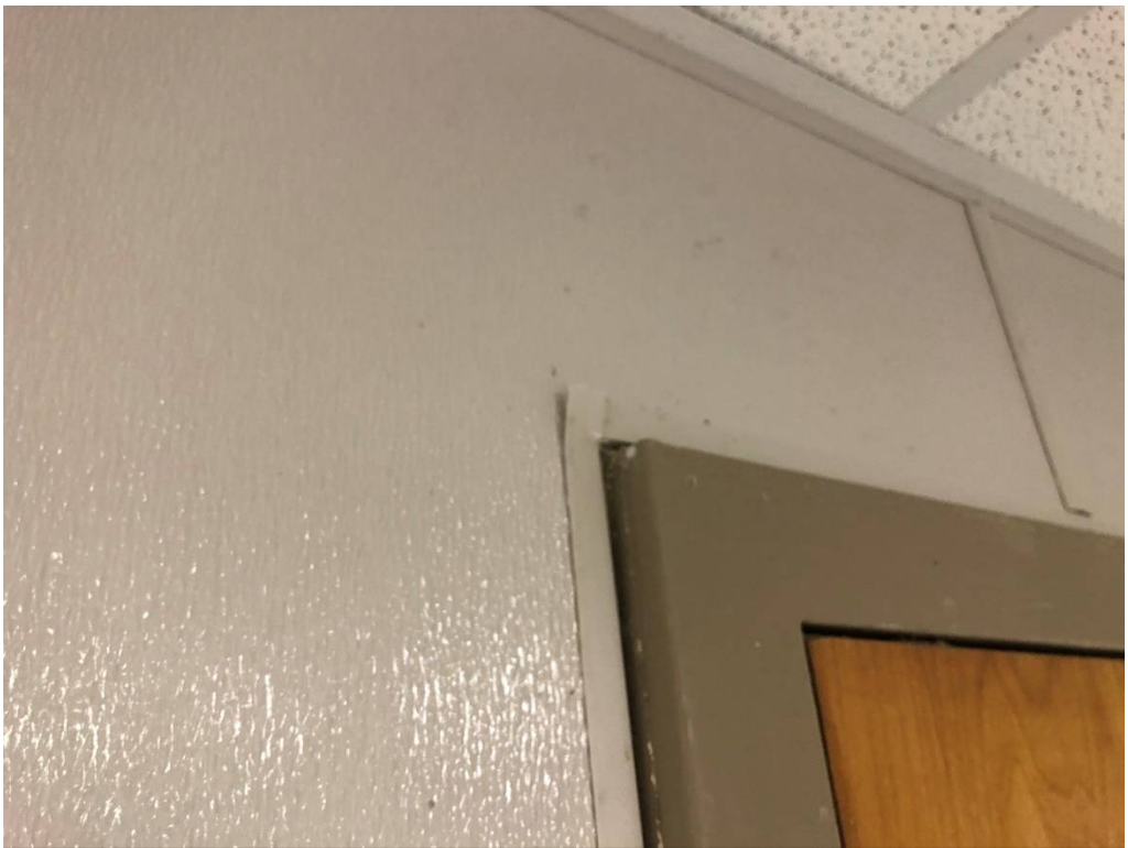
Figure 8 –Upper Corner FRP Kicked Up
