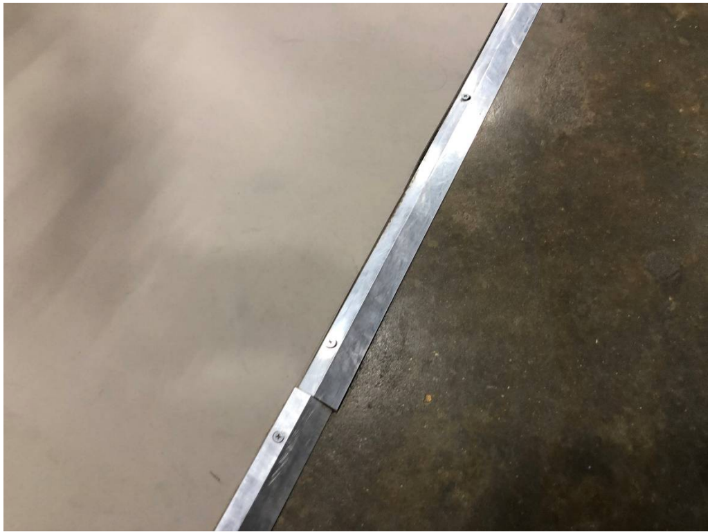
Figure 3 – Damage at Aluminum Threshold in Gym
