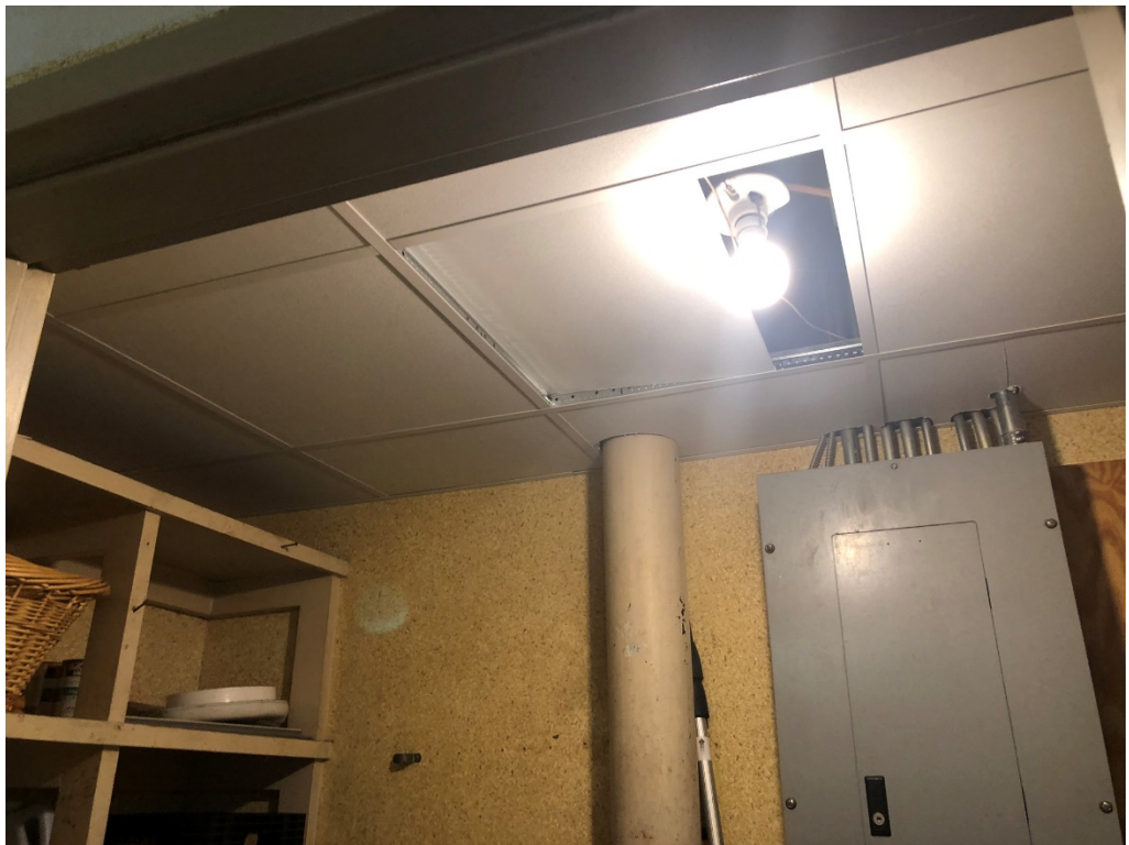
Figure 4 – Building 1 Janitor's Closet Ceiling
