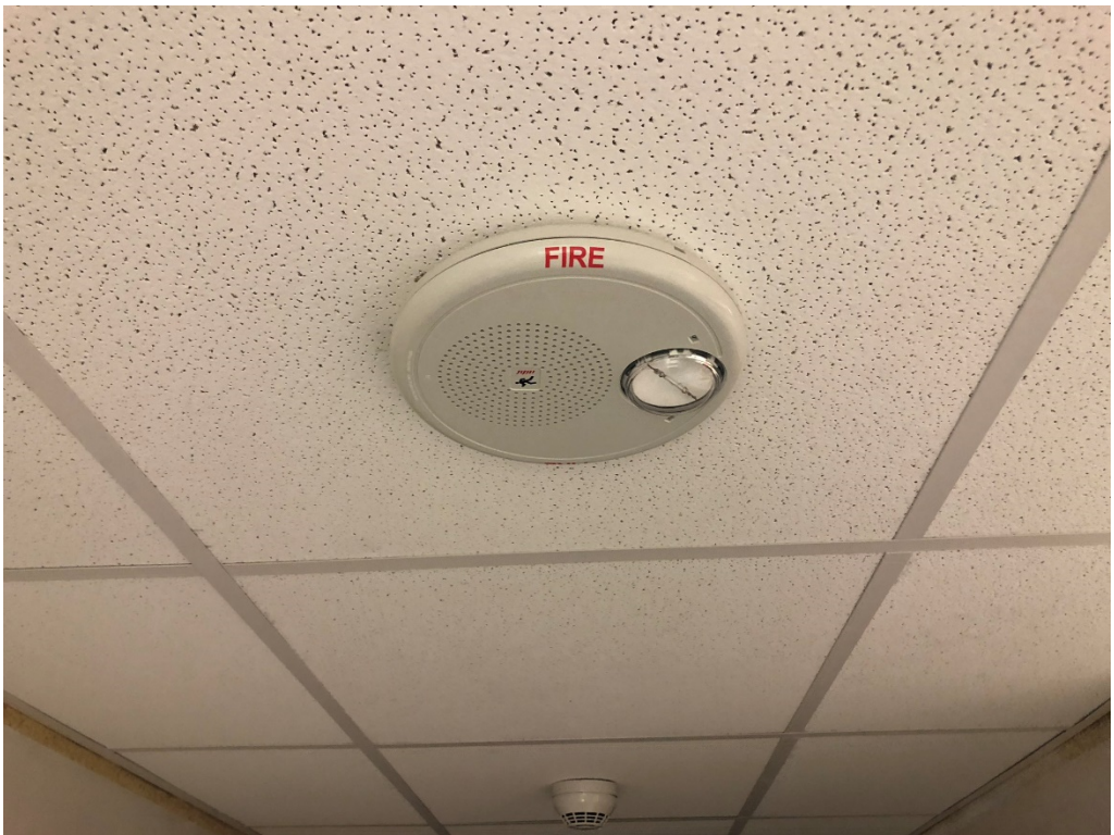
Figure 8 – Fire Alarm Installed in Vestibule Building 3
