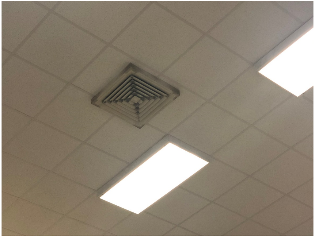
Figure 5 – High Ceiling Vents in Building 1
