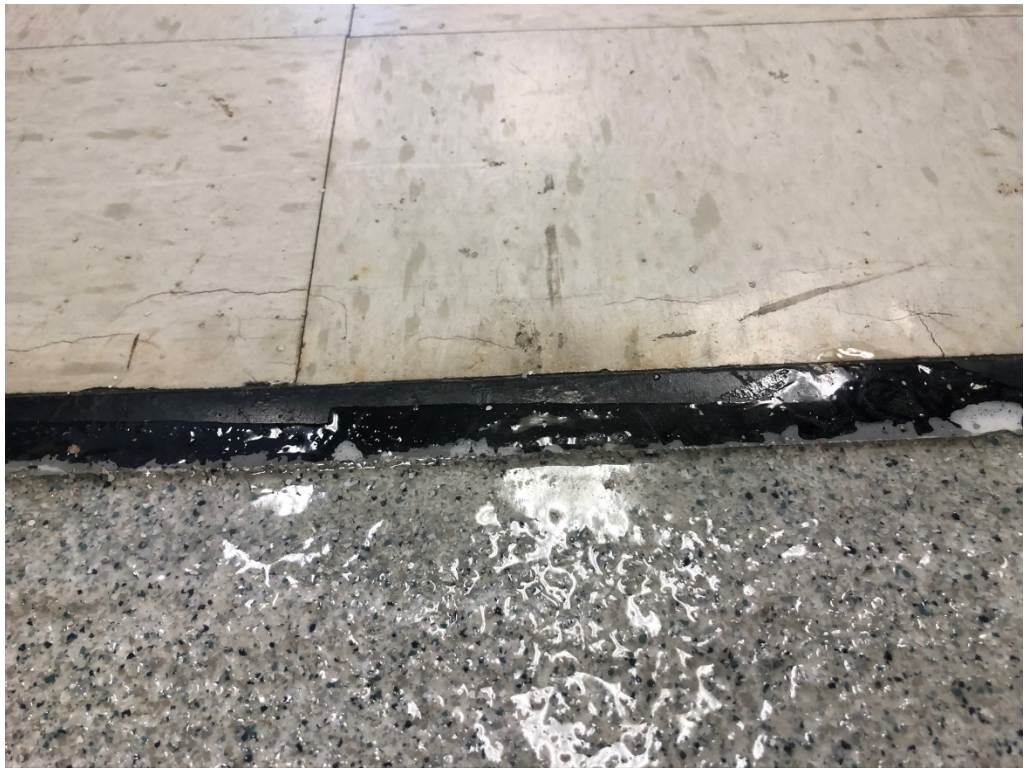
Figure 11 – Cleaning of Threshold Necessary
