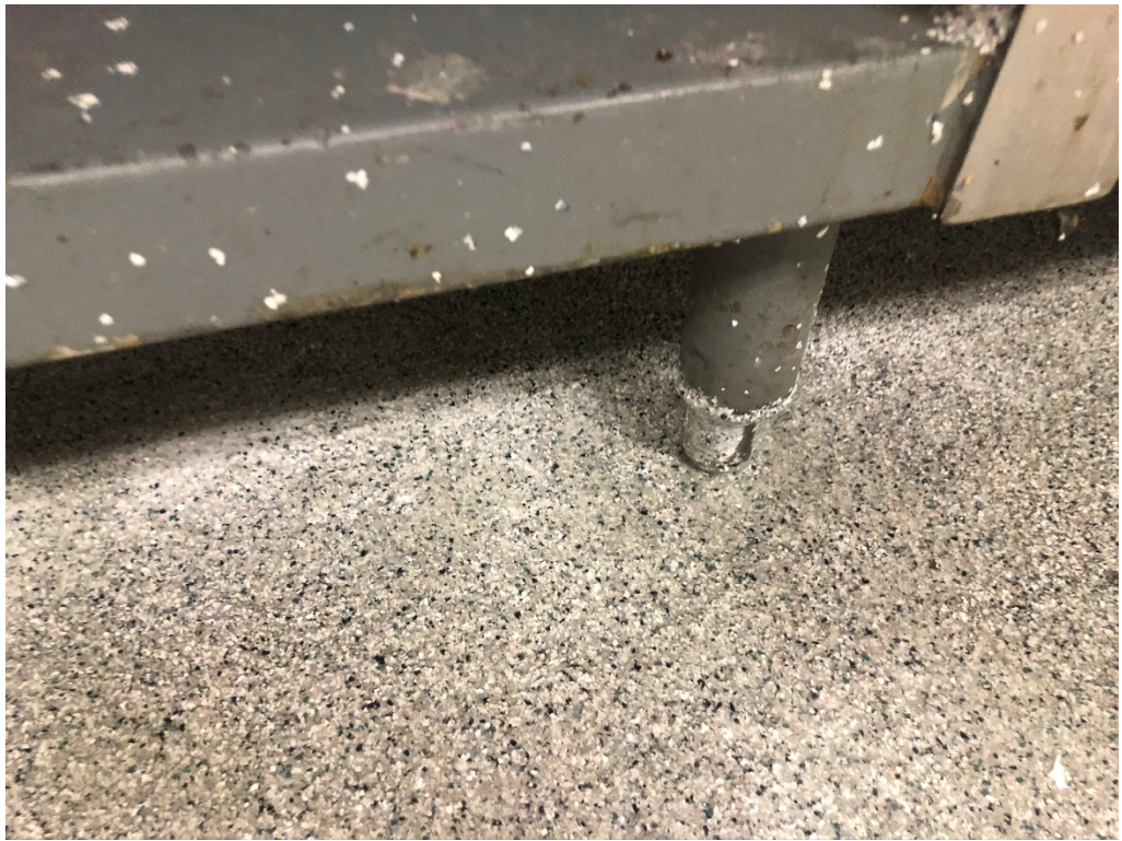
Figure 7 – Clean up Required @ Kitchen Equipment
