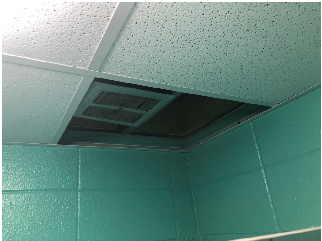
Figure 14 – Ceiling Tile and Vent Unfinished (RM T07)
