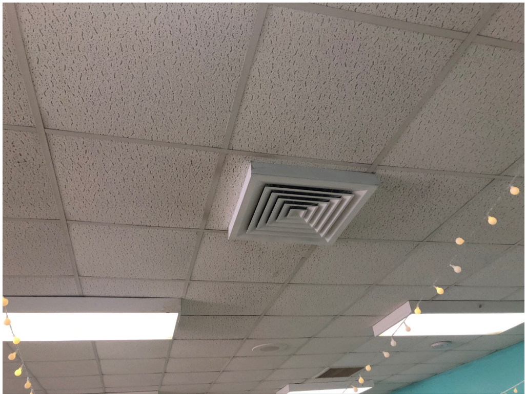
Figure 12 – Some Touch up Required at Paint for this Vent in Lobby A
