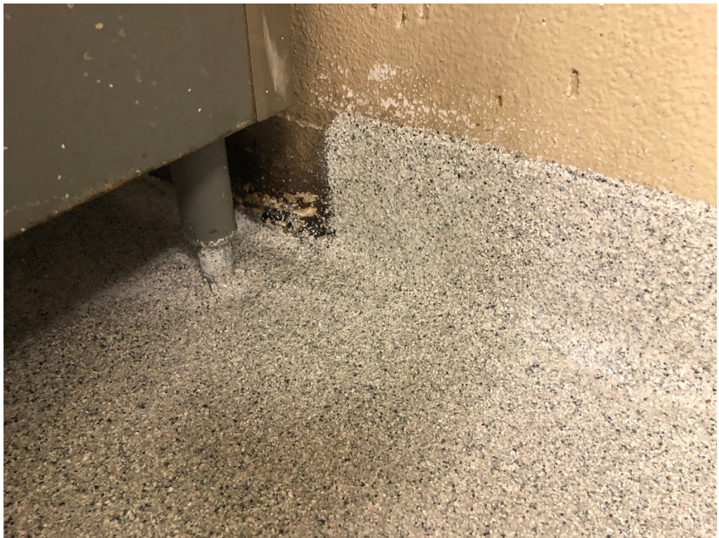
Figure 8 – Unfinished due to Inability to Move Kitchen Equipment
