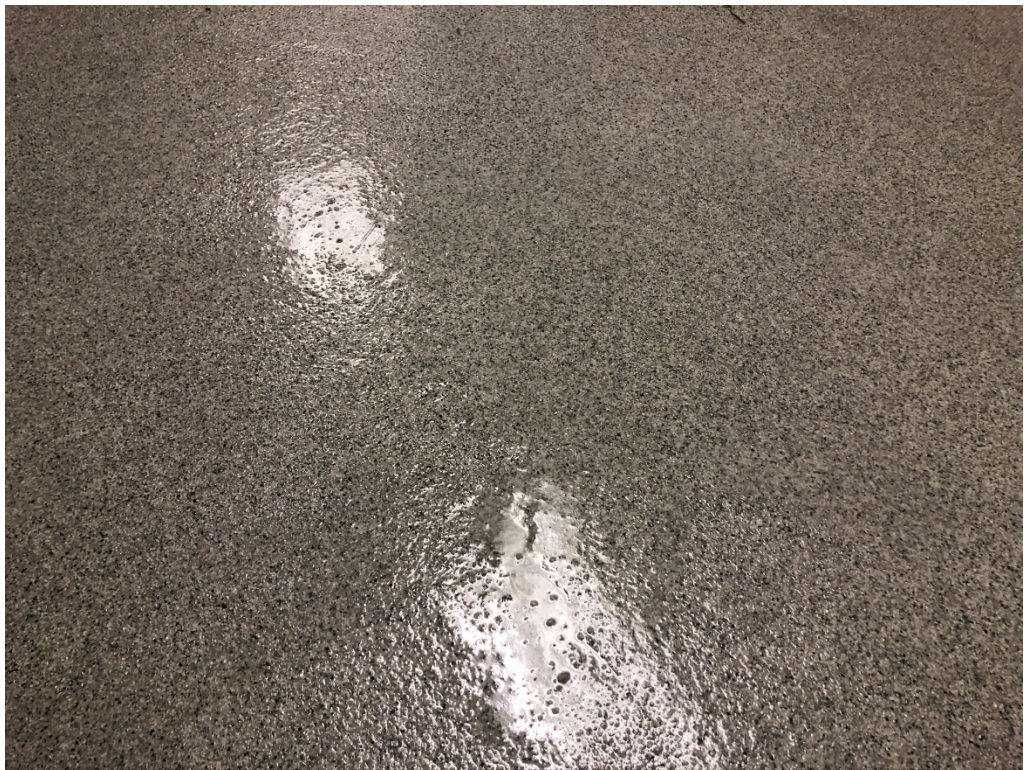
Figure 10 – Field Gloss Uneven (contractor indicated that they would add 2 nd coat to correct)
