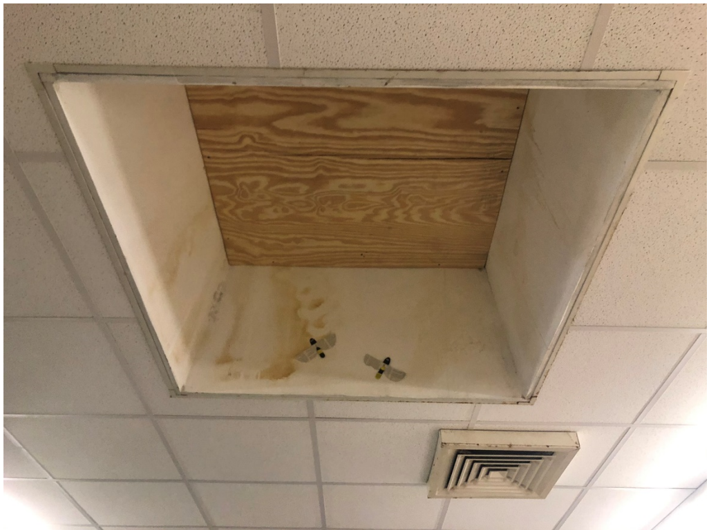
Figure 2 – Building 2 Art Class (rust on old grid)
