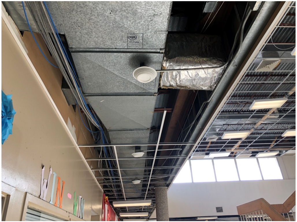
Figure 3 – Building 3 Corridor Supply Lines
