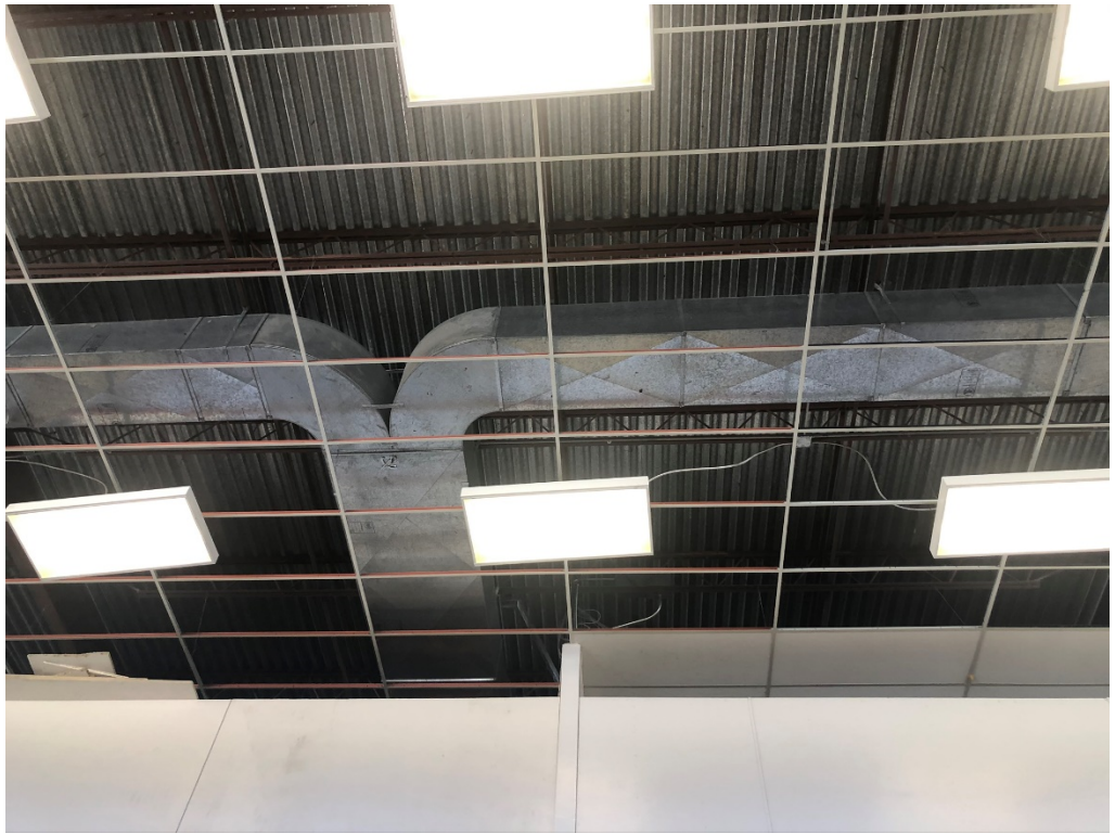
Figure 3 – Building 3 Corridor Supply Lines
