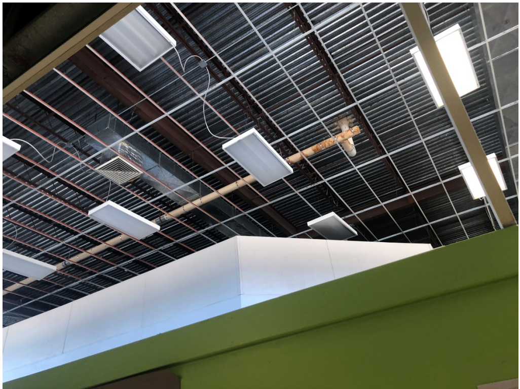
Figure 2 – Building 3 Corridor (Note Rust Stains on Roof Drain)
