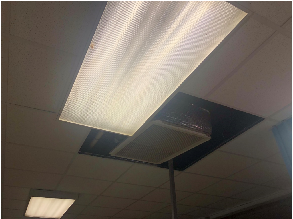
Figure 4 – Building 3 Cafeteria Unfinished Registers
