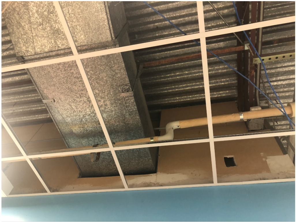
Figure 7 – Pipe Hanger Not In use
