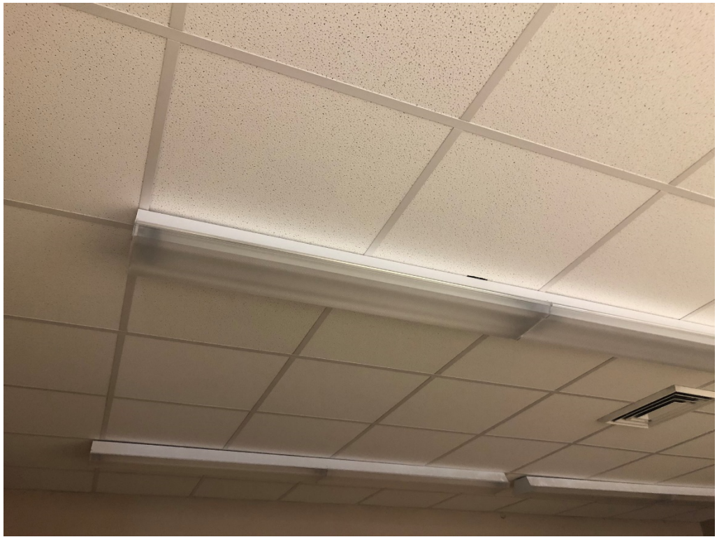
Figure 3 – Building 3 Cafeteria Notch Showing @ Light
