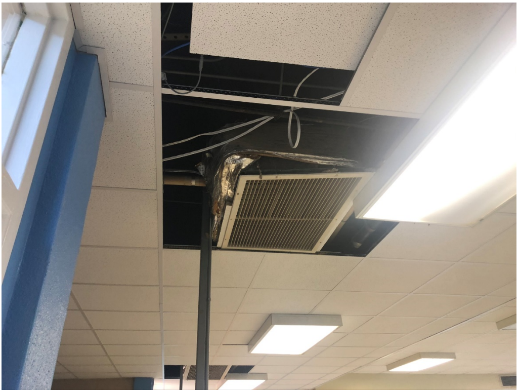
Figure 2 – Building 3 Cafeteria Unfinished Registers
