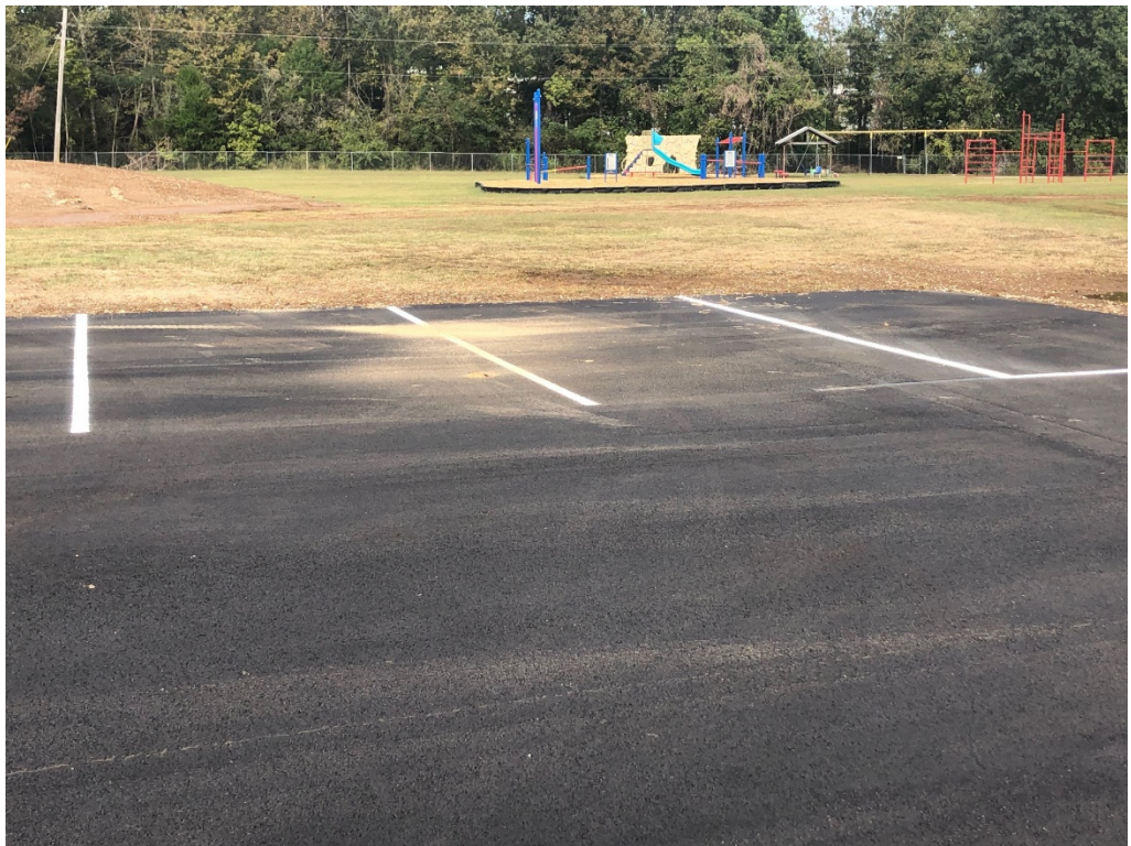
Figure 4 – Low Spot in Asphalt
